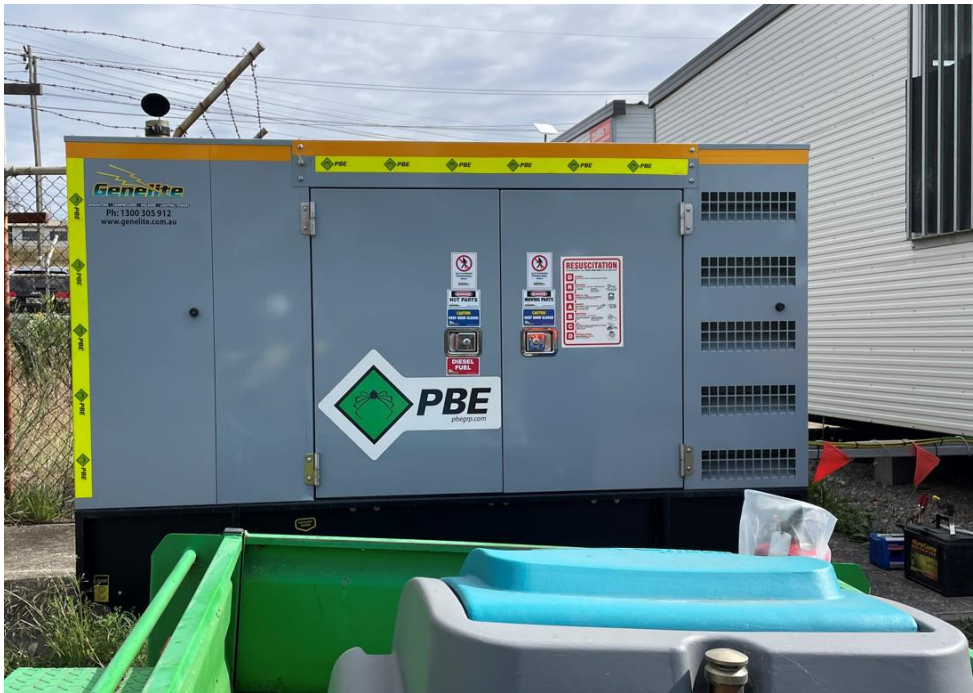
Plate 1 Bunded diesel storage area at project laydown area
