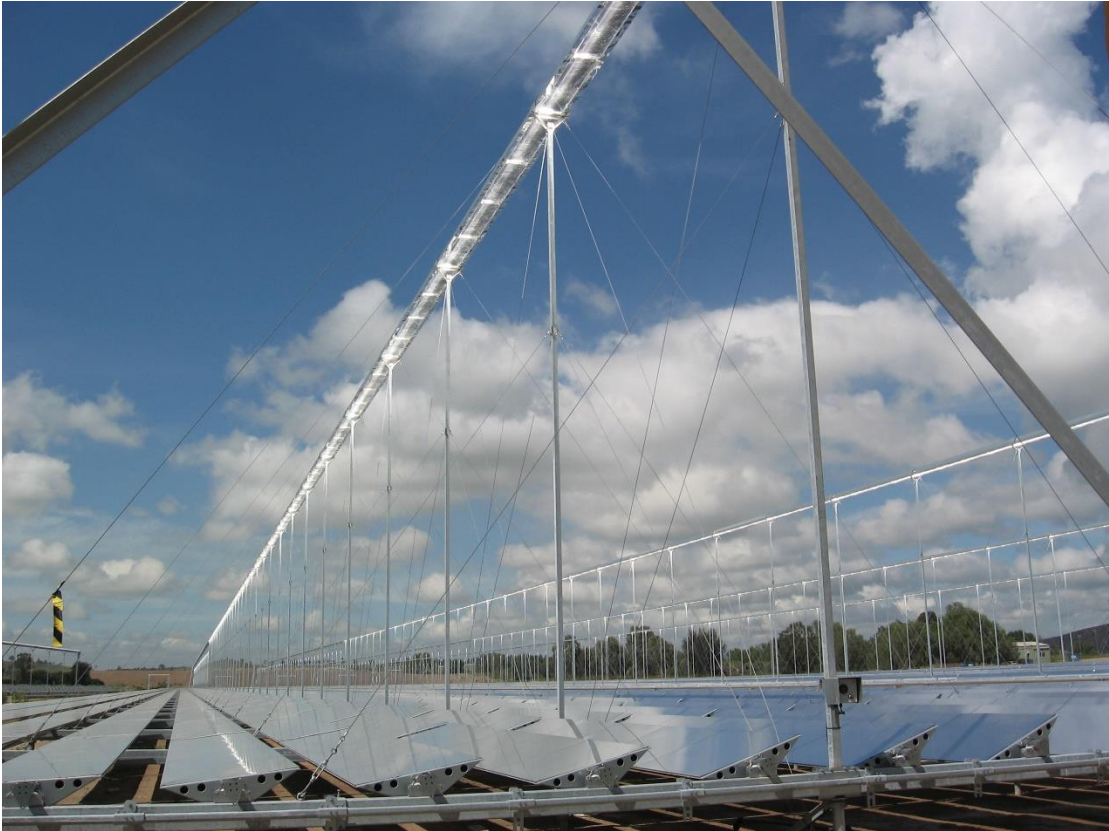
Figure 2 Existing solar array area
