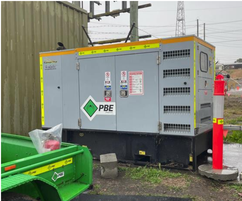
Plate 1 Bunded generator area at project laydown area
