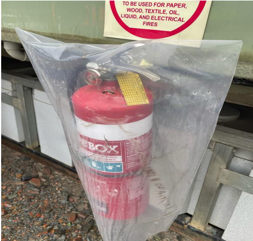
Plate 7 Tagged portable fire equipment available at project laydown area
