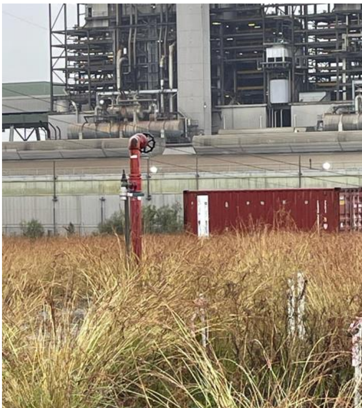
Plate 12 Hydrant used as site water source
