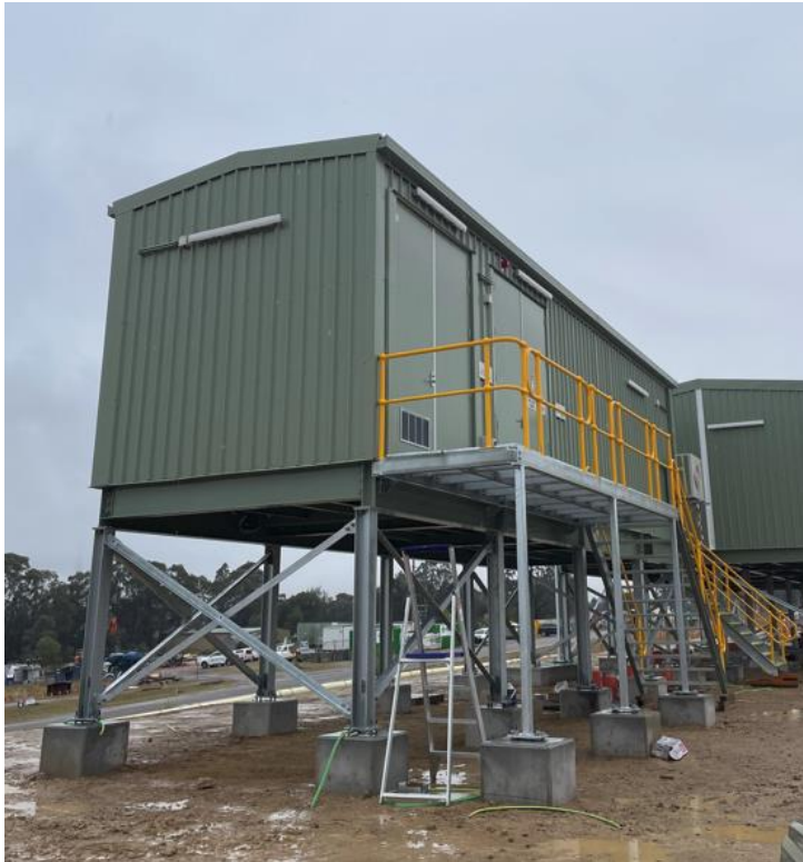
Plate 11 External lighting on project building
