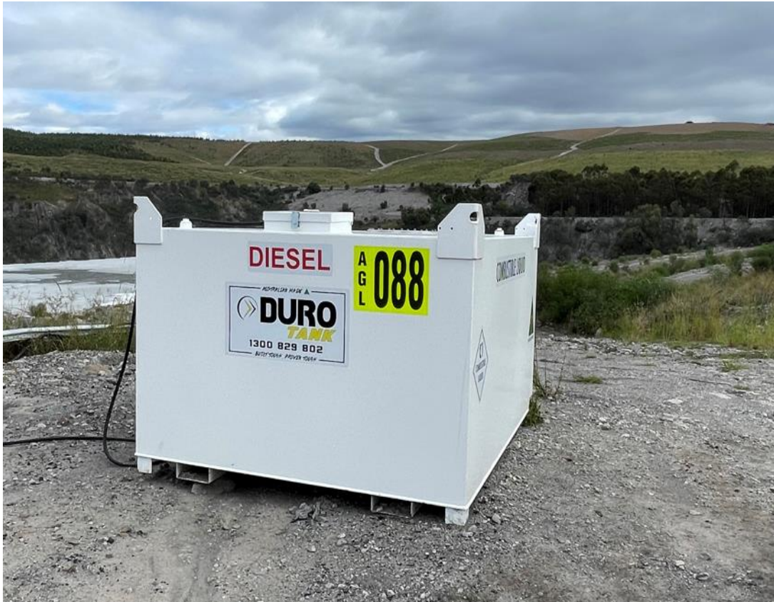
Plate 7 5000 L Diesel secondary containment tank available on site
