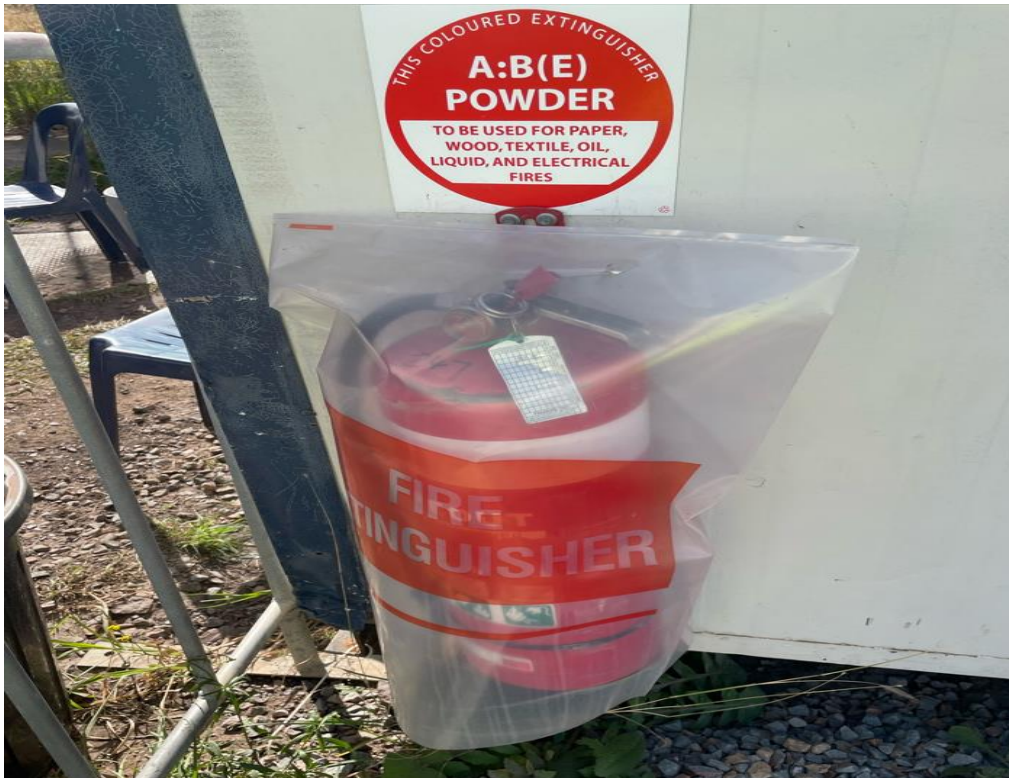
Plate 5 Firefighting equipment available at the project construction offices and in good condition
