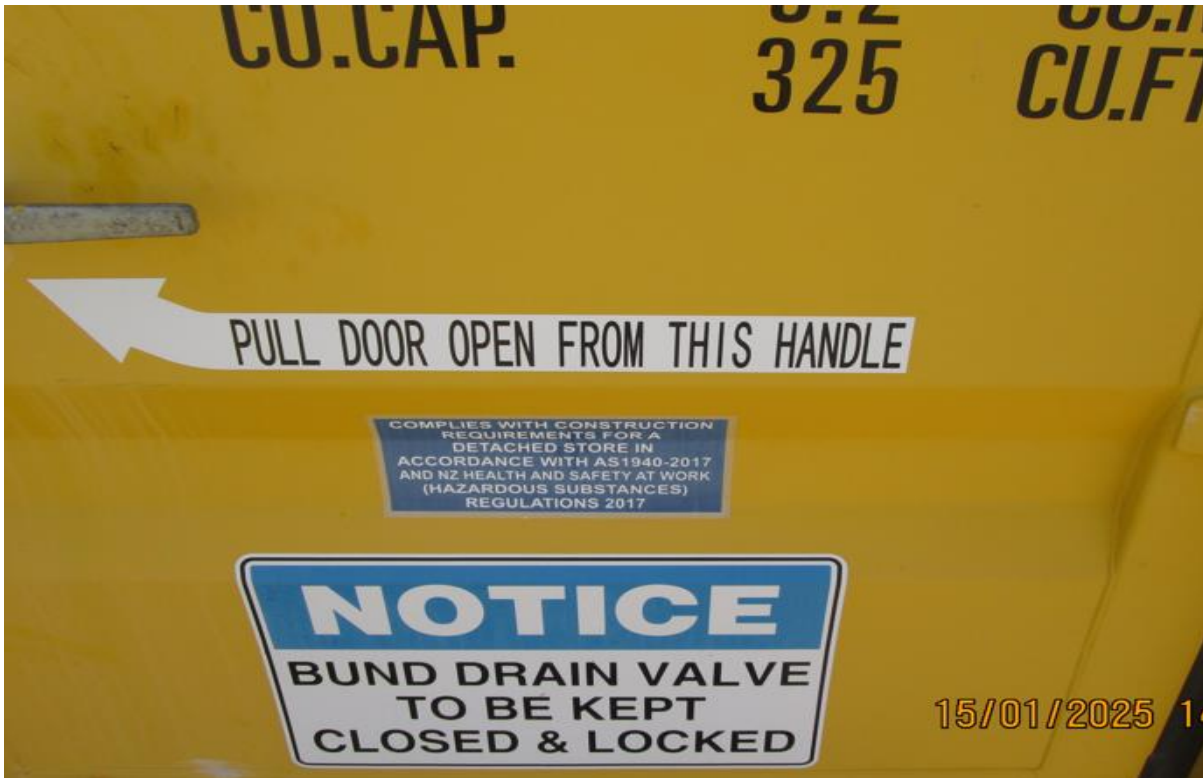
Plate 9 – Bunded chemical storage in accordance with AS 1940-2017
