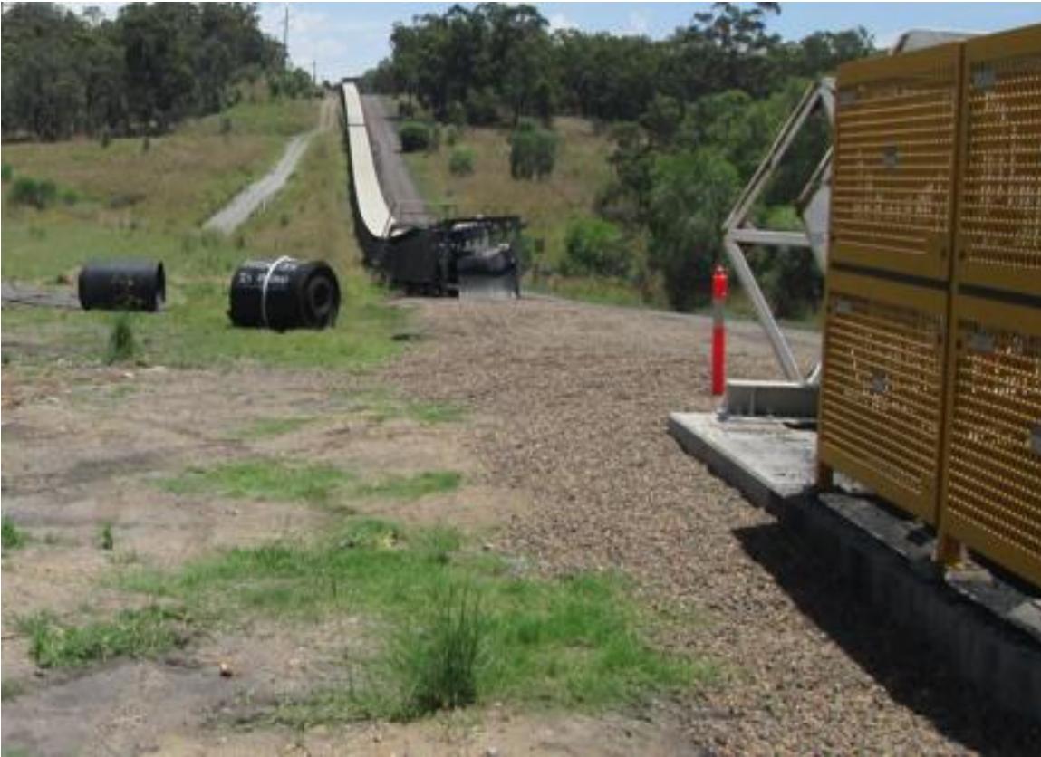
Plate 13 – Deconstructed section of Liddell MA1B conveyer completed under Project Stage 3 during the audit period
