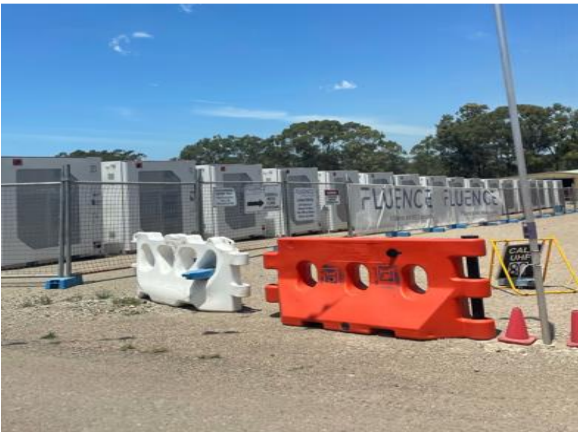
Plate 16 – Fenced off battery storage area for Stage 2
