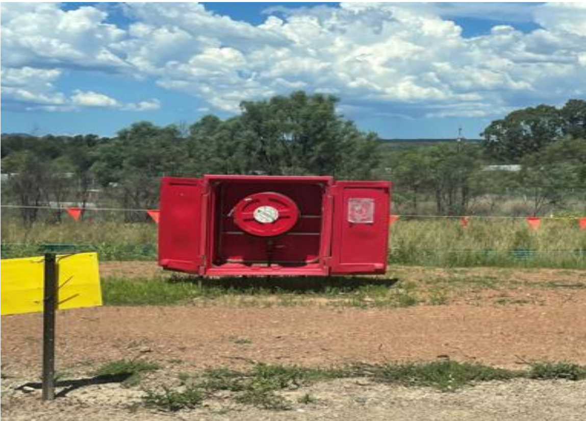
Plate 14 – Fire fighting equipment available for Stage 3 of the Project
