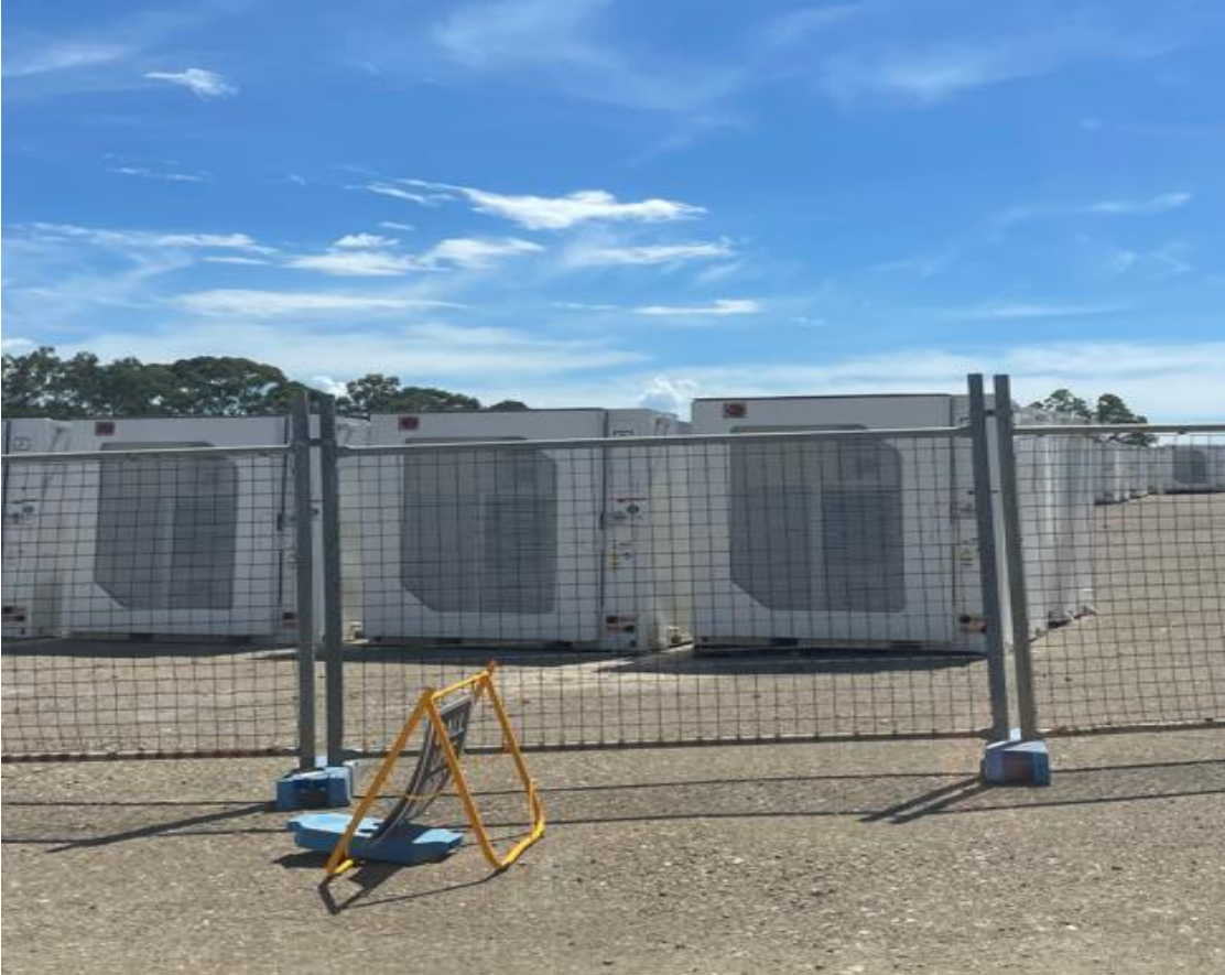
Plate 17 – Fenced off battery storage area for Stage 2
