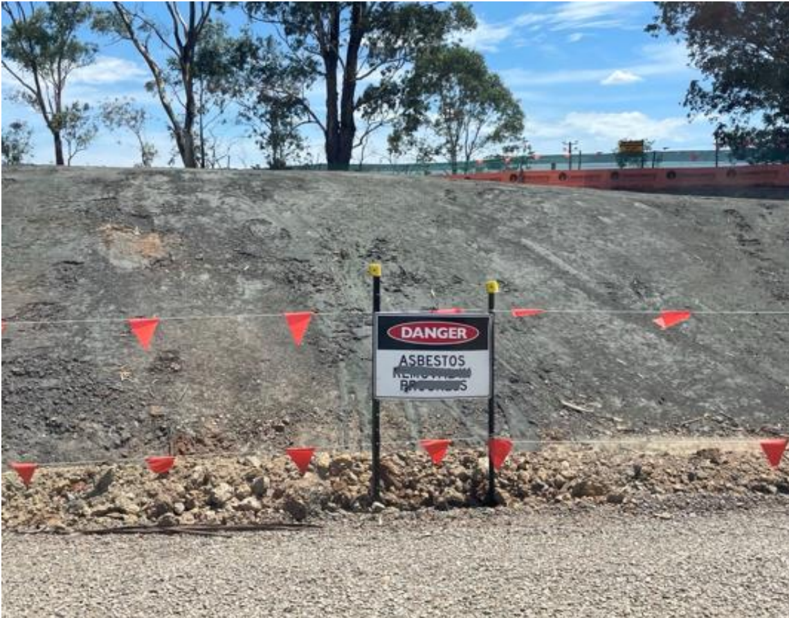
Plate 15 – Signed and flagged stockpile with contaminated Asbestos materials identified for Stage 2
