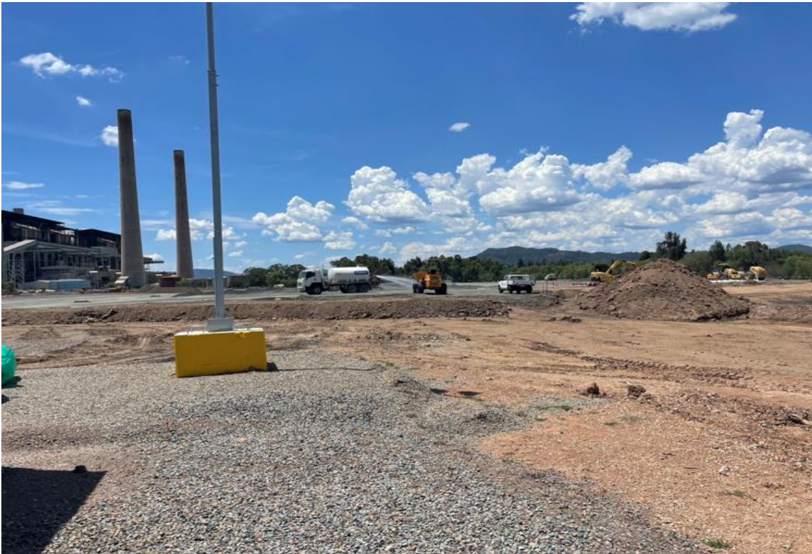
Plate 1 - Water cart being used for dust suppression within the Stage 2 construction area
