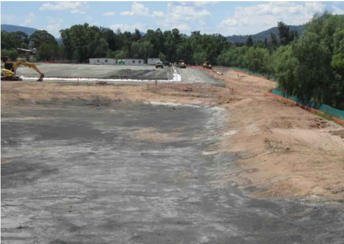
Plate 10 – Stage 2 Project site being maintained in a good condition with sediment fencing in place and low dust emissions
