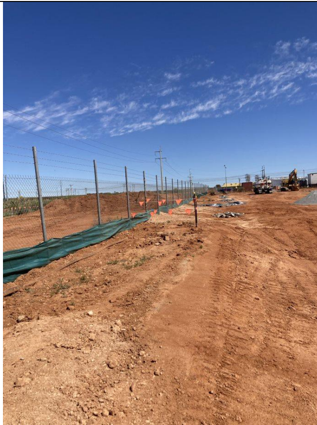
Photograph 11 Non-compliant soil stockpile outside construction pad boundary.
