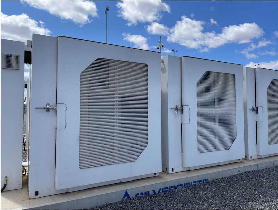
Photo C9: Fluence Energy Gen 6 Cube (battery enclosure) system
