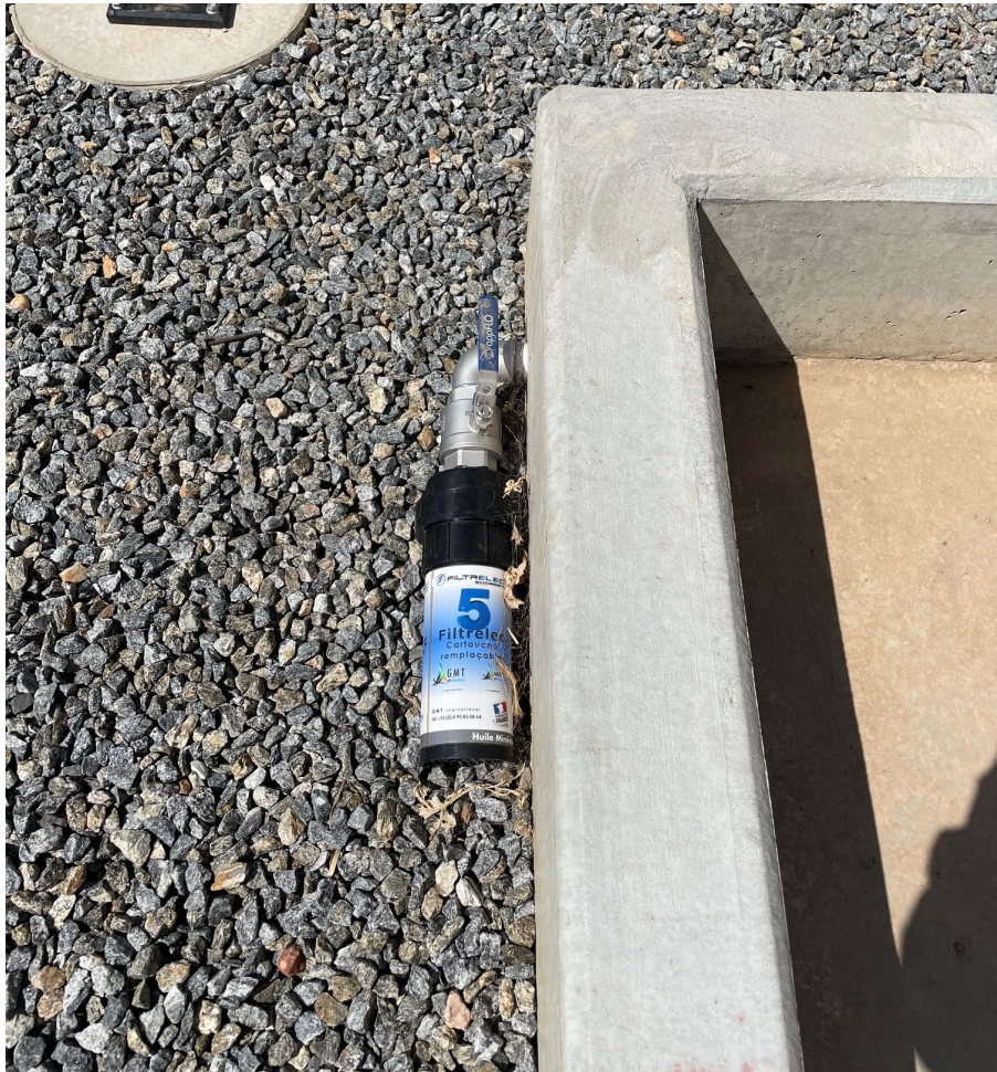
Photo C7: Transformer bund with water treatment (carbon filter)
