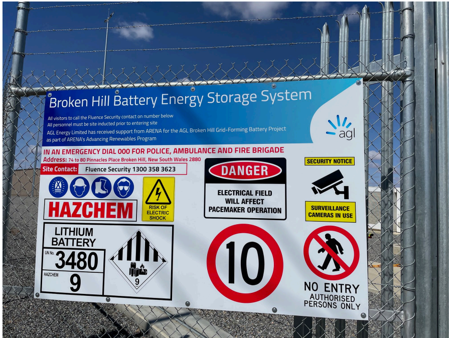
Photo C1: Broken Hill Battery Energy Storage System site signage
