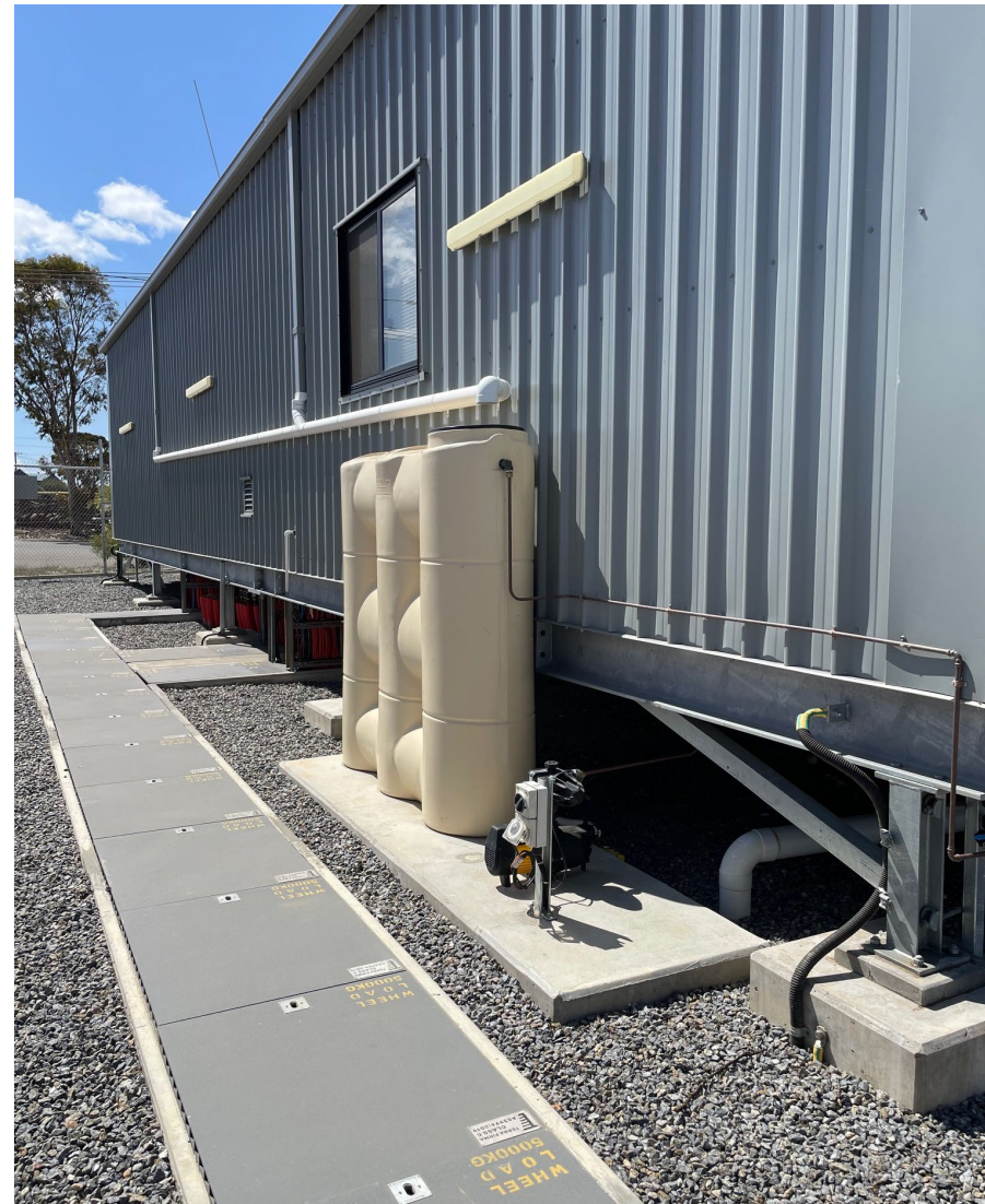
Photo C6: Control Building water tank
