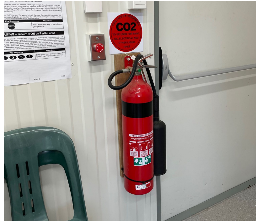
Photo C4: Control Building fire extinguisher
