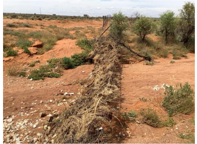
Plate 20: Damaged fence observed in 2020
