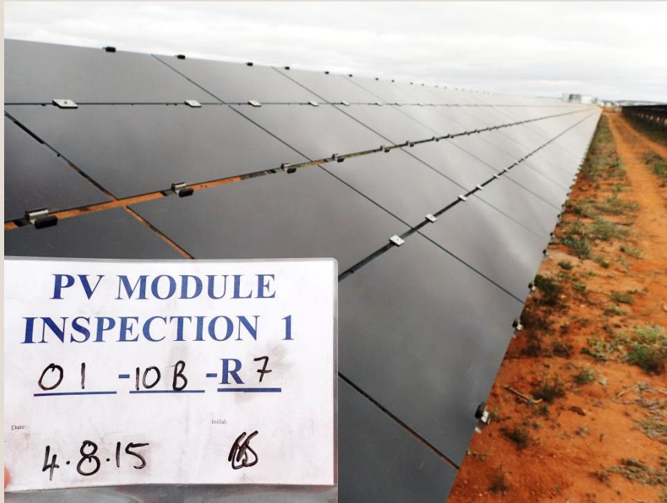
Quality inspection – solar panels
