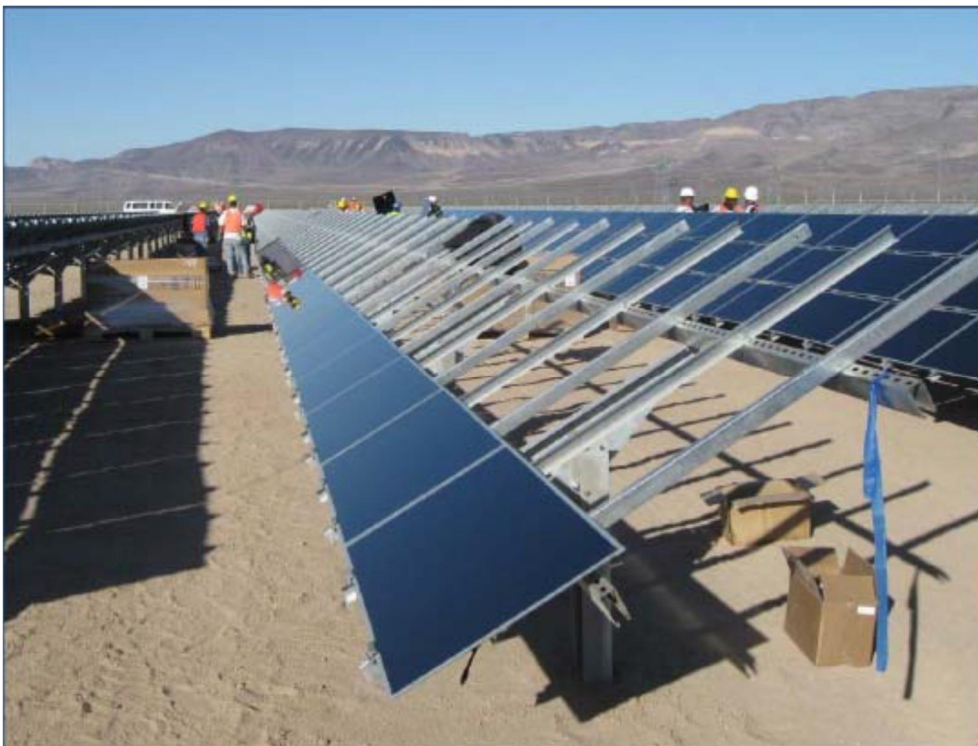
Figure 2 Example of solar modules and racking tables
