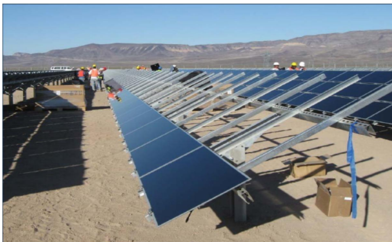
Figure 4-3 Example of solar modules and racking tables
