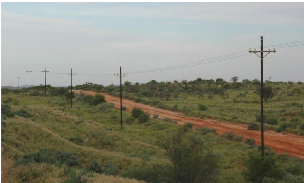
Figure 5-4 Existing 22kV transmission line near the site
