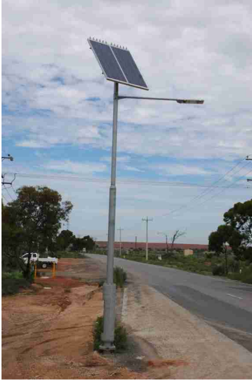
Figure 12 Street lighting powered by solar panels on Kanandah Road.
