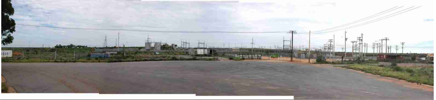
View west toward Transgrid Broken Hill substation
