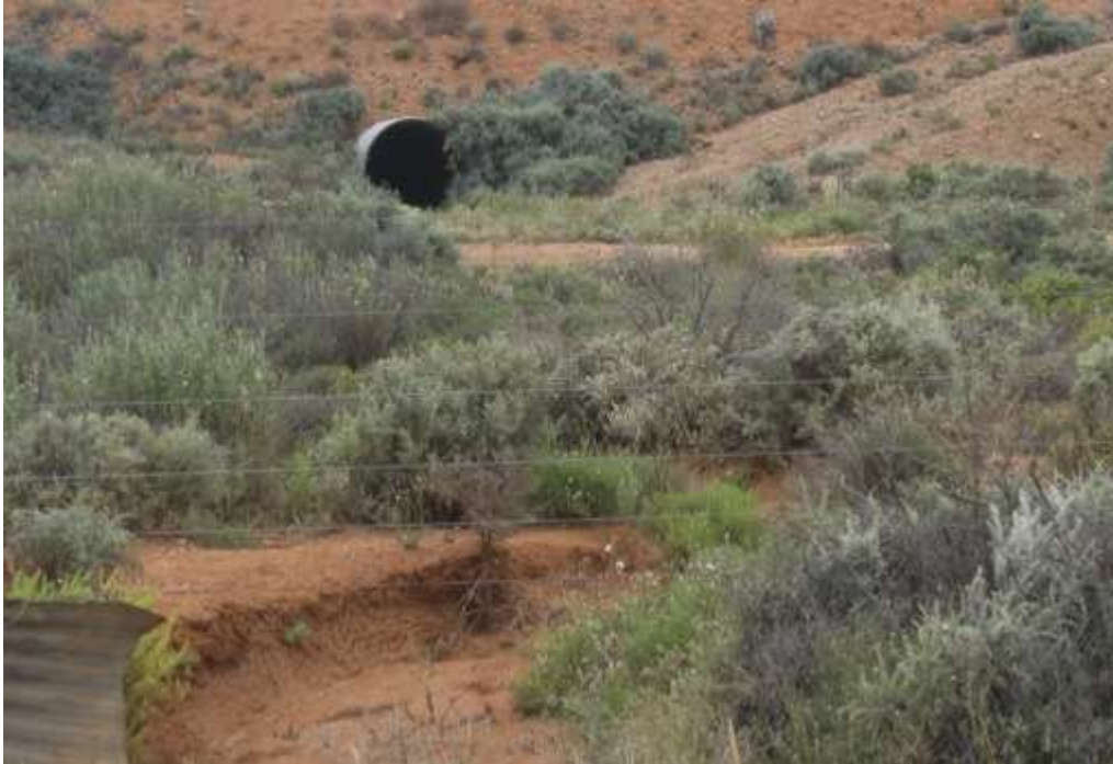
Plate 11: The culvert beneath the Port Pirie to Broken Hill Railway line. The fence in the foreground marks the southern boundary of the study area. Note the potential for the ephemeral channel to increase in width and depth as the metal piping within the culvert concentrates and diverts water along the drainage channel. (Image, M. Cotter).
