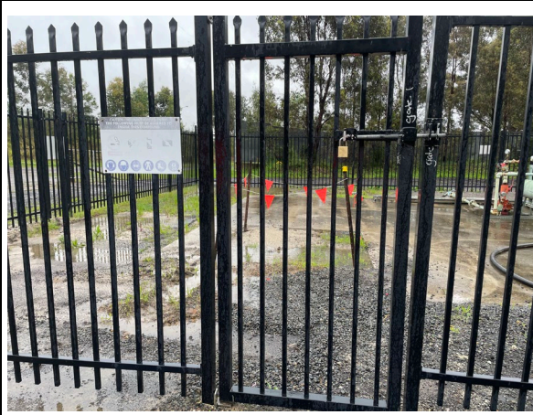
Photo 7: Well site SF5 (decommissioned). Well site SF5 is co-located with well sites SF07 and SF08 which are operational
