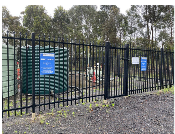
Photo 8: Well sites SF07 and SF08 (operational)
