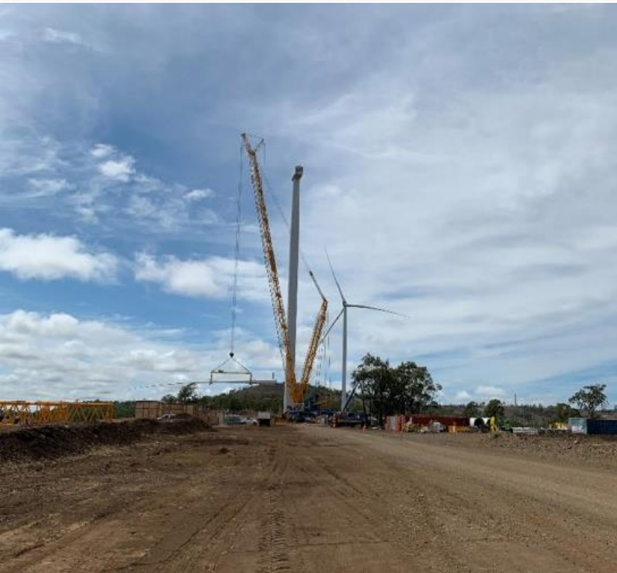
Coopers Gap Wind Farm | 13 March 2019
