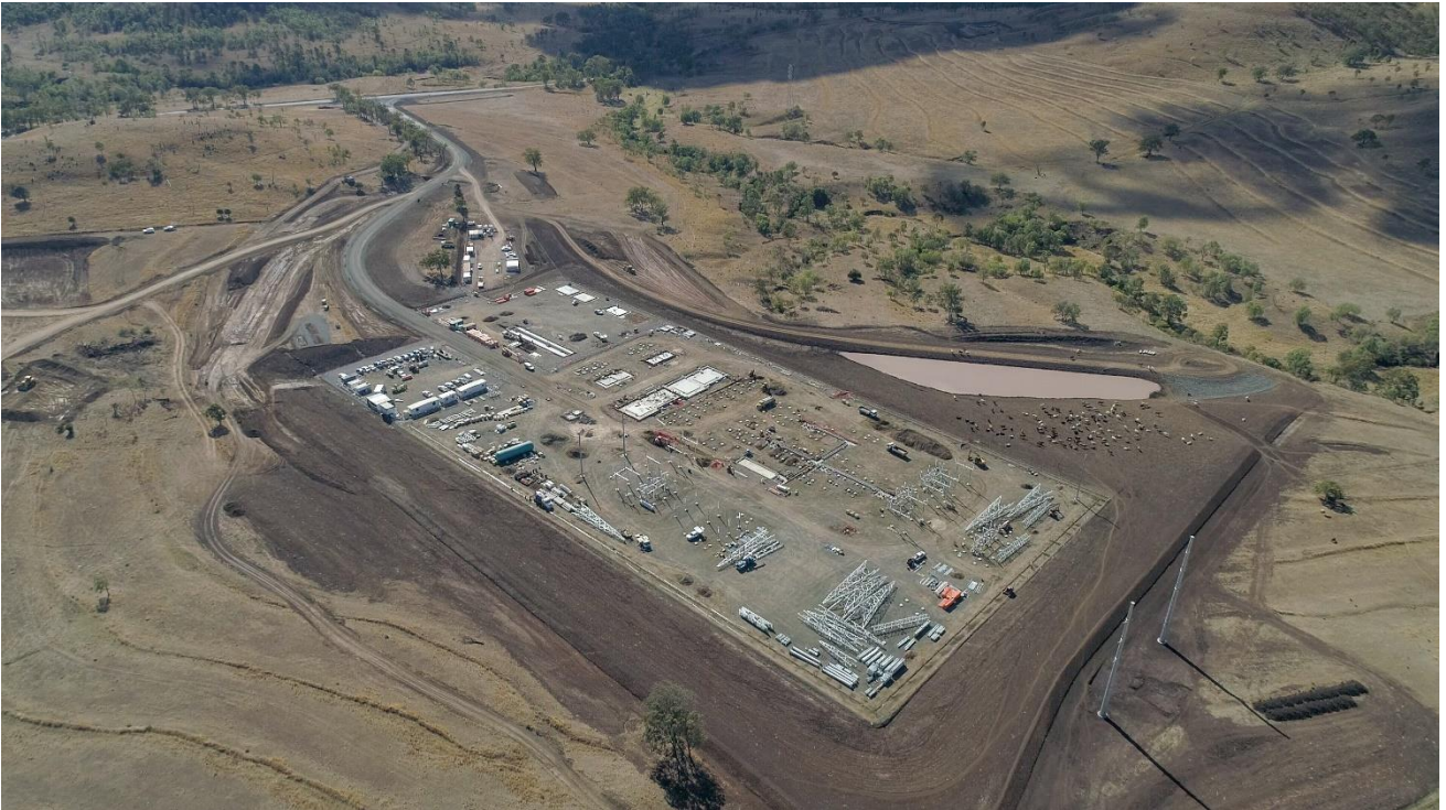
Aerial view of the substation area Coopers Gap Wind Farm is owned by the Powering Australian Renewables Fund (PARF). All images courtesy of PARF.
