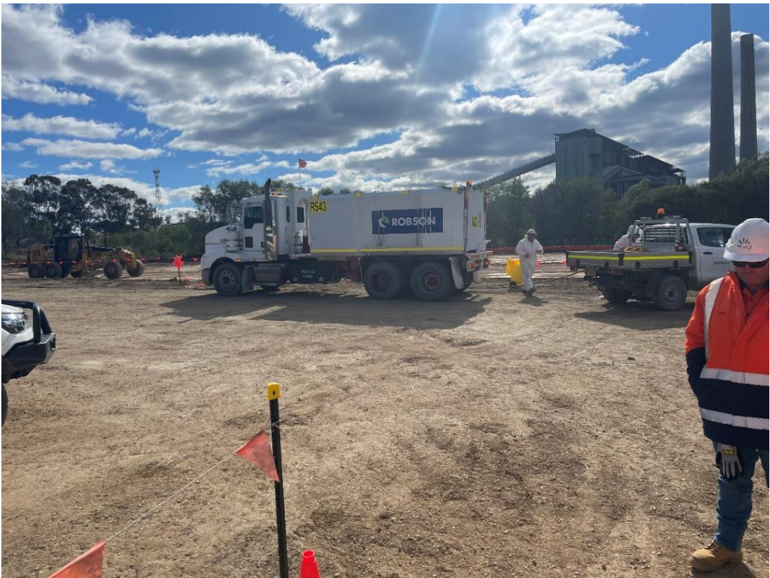
Plate 4 Mobile truck refuelling equipment in the Stage 2 area
