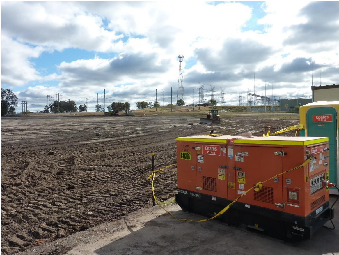
Plate 1 Area 1, Stage 2 disturbance preparing area for BESS installation Note: Completed Stage 1 facilities in the background
