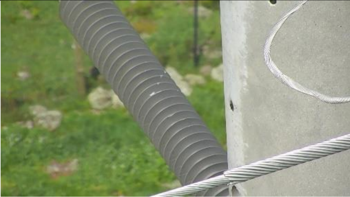
Damaged insulators (minor) picked up through inspections identified and captured in the replacement program (2020).
