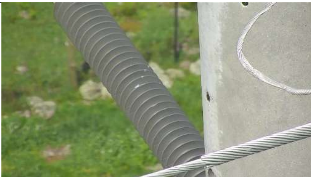
Damaged insulators (minor) picked up through inspections identified and captured in the replacement program (2020).
