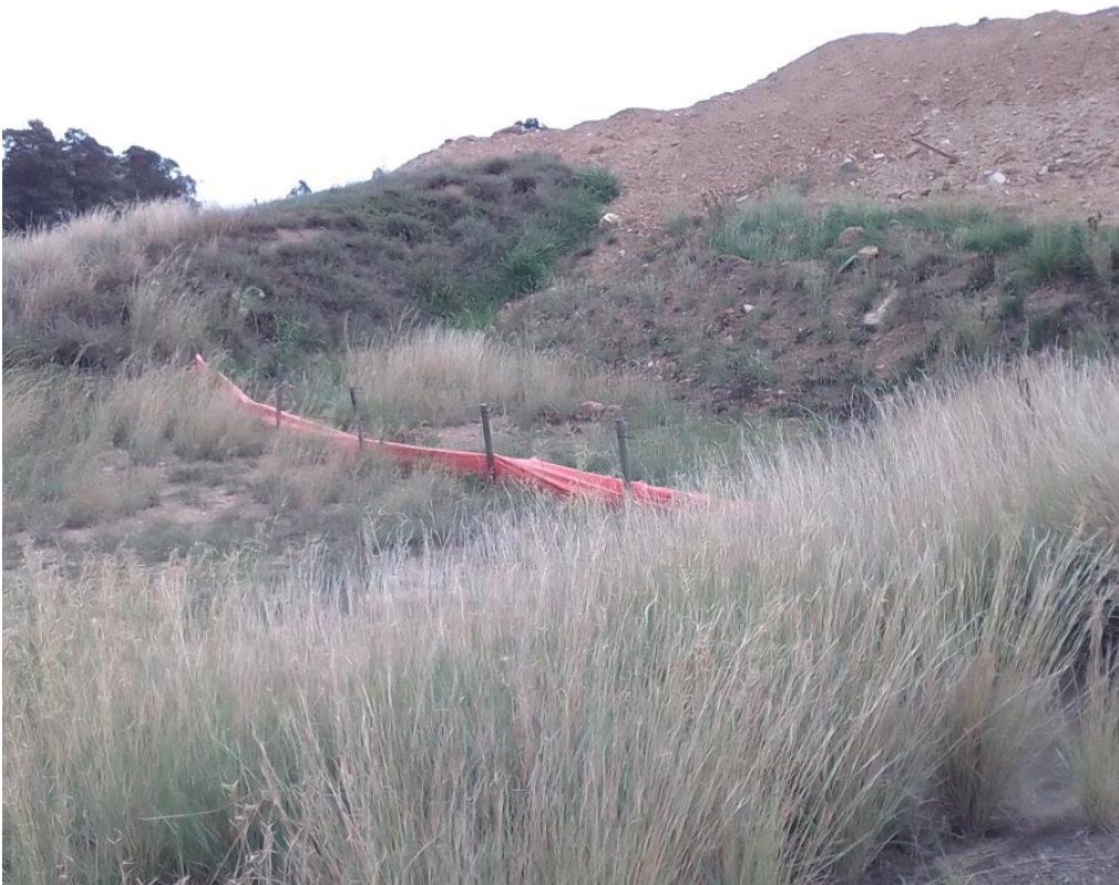
Plate 2 Stage 1 sediment fencing that requires maintenance while stockpile is exposed
