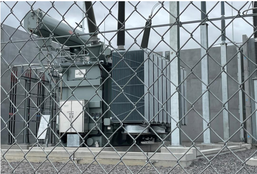
Plate 6 Stage 1 transformers with bunding available to capture any spills
