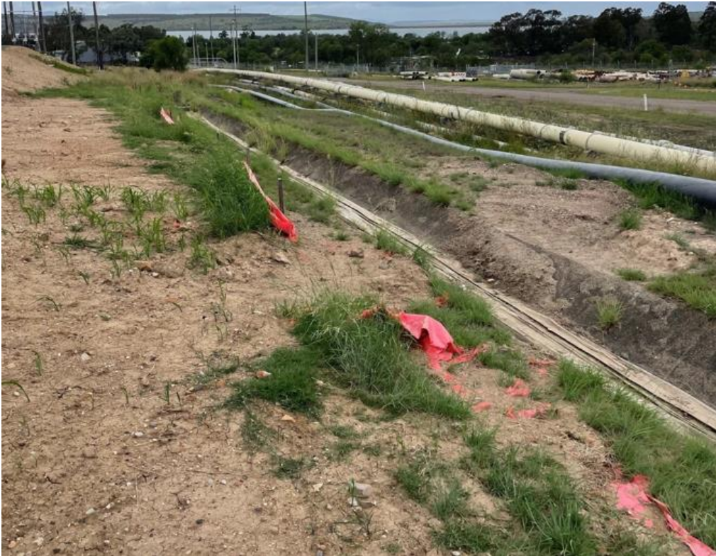
Plate 1 Sediment fencing requiring maintenance on the Stage 1 site while ground cover develops
