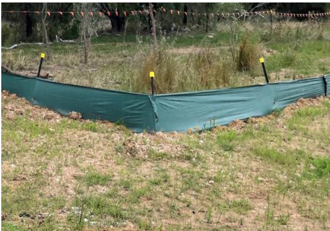
Plate 16 Sediment fencing available within the Stage 2 site used to define clearing area
