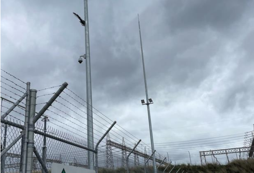
Plate 7 Lighting at Stage 1 facility positioned facing below horizontal
