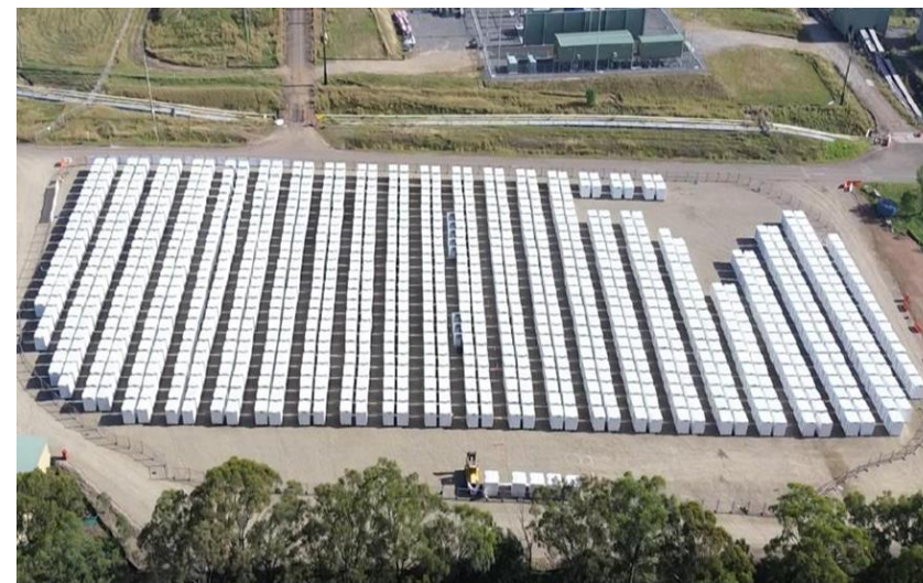
1,055 battery cubes delivered to the Liddell Battery layout area
