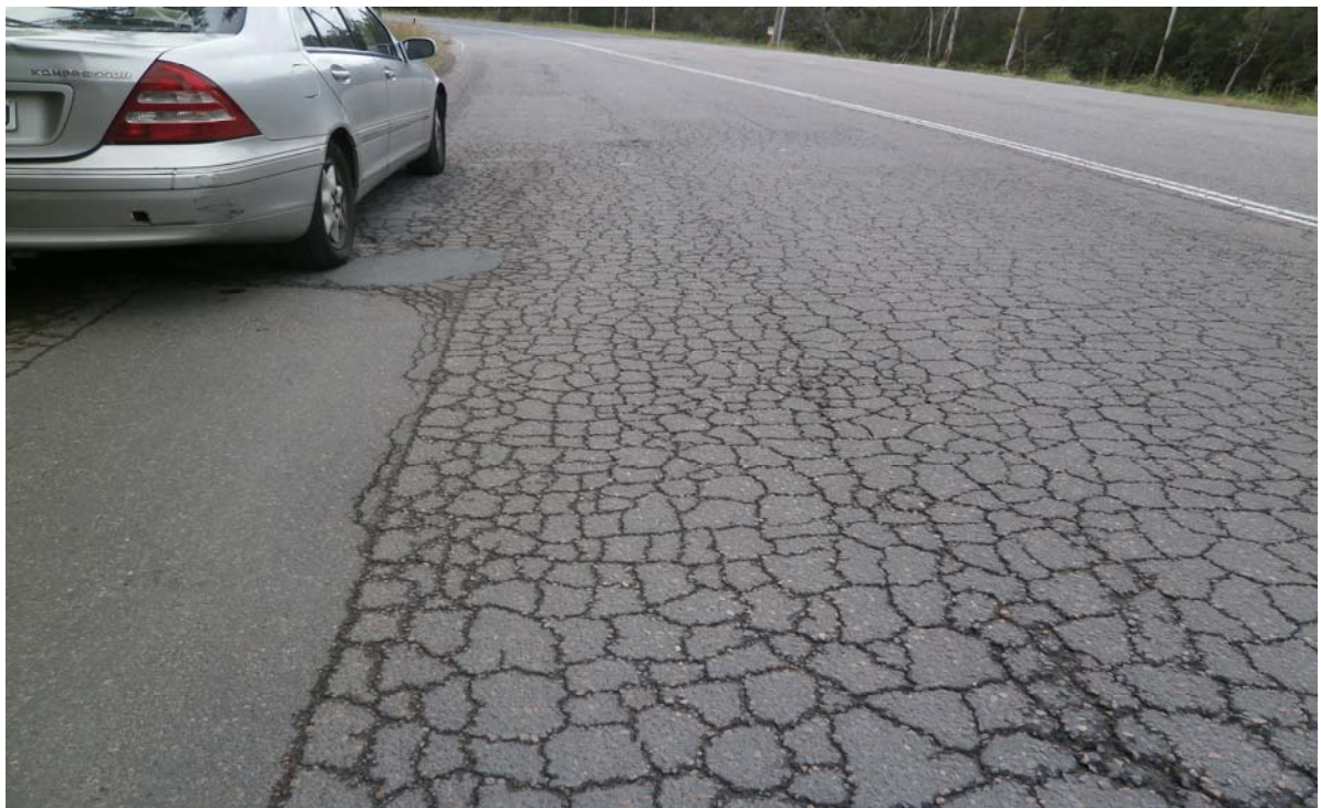
PHOTO P12 CROCODILE CRACKS IN BOTH LANES | OLD PUNT ROAD FOR 256.6M WEST OF NORTHERN SMELTER ACCESS ROAD. (TAC) Ch 1720 TO Ch 1975 (Sheet 13/19)
