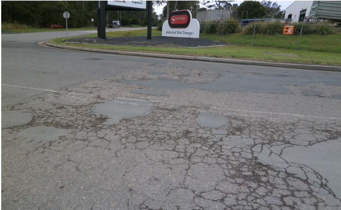
PHOTO P9 CROCODILE CRACKING IN PAVEMENT IN OLD PUNT ROAD CH 130.0 SOUTH OF SPEEDWAY ROAD TO INDUSTRIAL PARK. Ch 2850 (Sheet 9/19)
