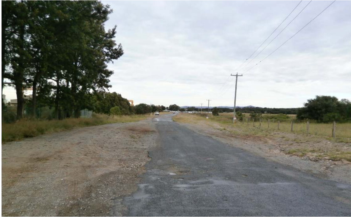
PHOTO P5 VIEW SOUTH OF PRIVATE ROAD TO FORGACS. PAVEMENT POOR CONDITION FOR 50 METRES. UNCHANGED SINCE 11-12-13.
