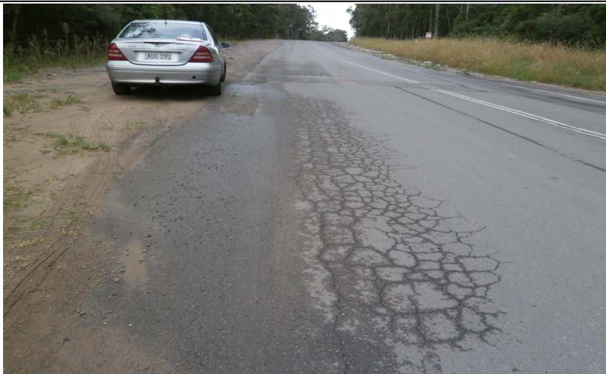
PHOTO P10 CROCODILE CRACKING IN OLD PUNT ROAD CH 2610 (Sheet 10/19) NORTH OF KENNINGTON DRIVE AT END OF KERB AND GUTTER.
