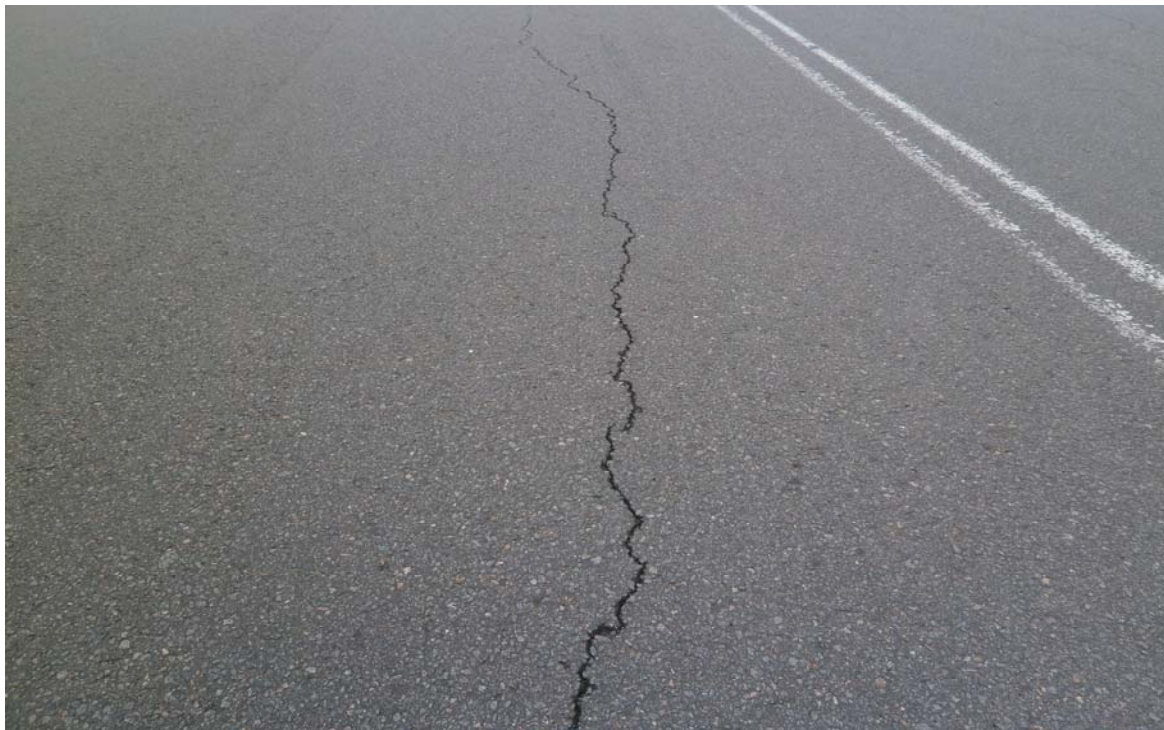
PHOTO P8 TYPICAL LONGITUDINAL CRACK IN ASPHALT NEAR EXIT DRIVEWAY FROM KOMATSU. THESE CRACKS WERE EVIDENT IN DECEMBER 2014. Ch 3275
