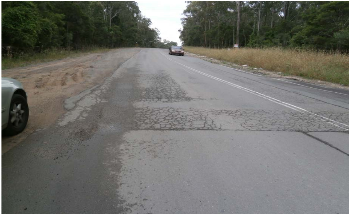
PHOTO P11 TYPICAL CROCODILE CRACKING 2.5 METRES FROM EDGE OF BITUMEN IN OLD PUNT ROAD NORTH FROM CH 2599
