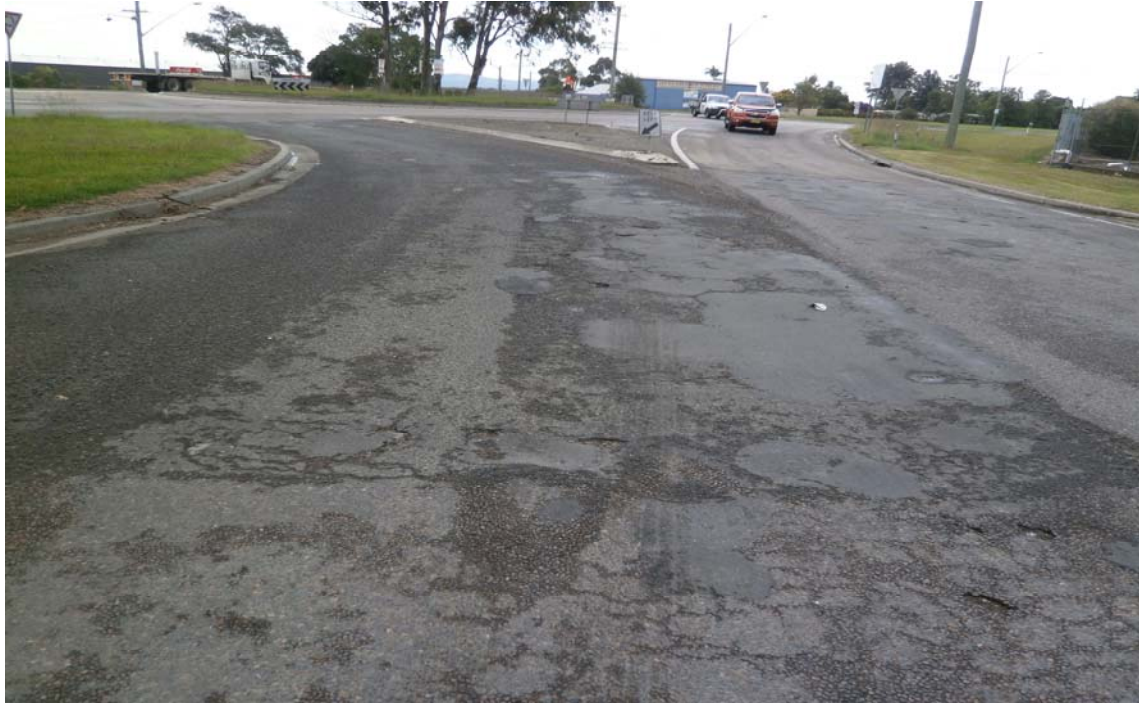
PHOTO P7 PAVEMENT POOR CONDITION NORTHERN APPROACH TO ROUNDABOUT IN OLD PUNT ROAD. Ch3602 to Ch3635
