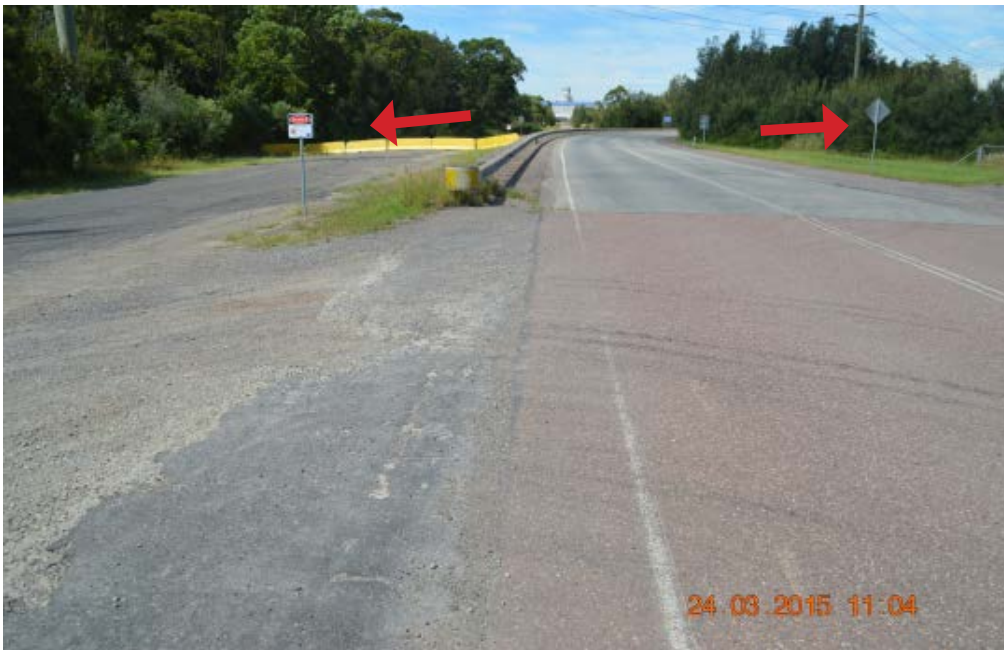
North side of Old Punt Road at 530 metres from the intersection with the Pacific Highway.
