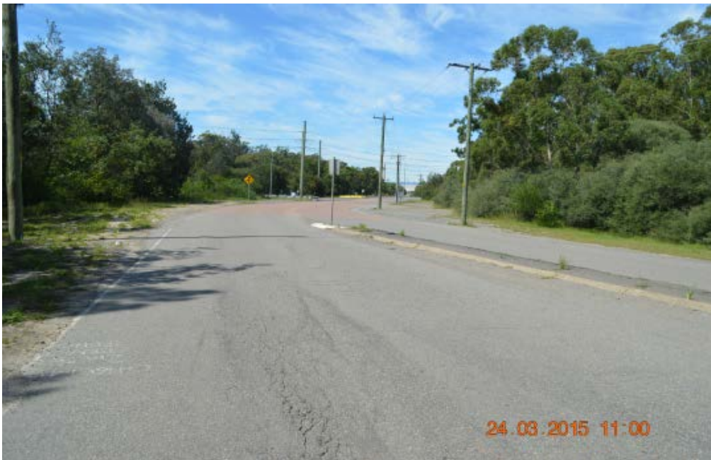
North side of Old Punt Road at 350 metres from the intersection with the Pacific Highway.
