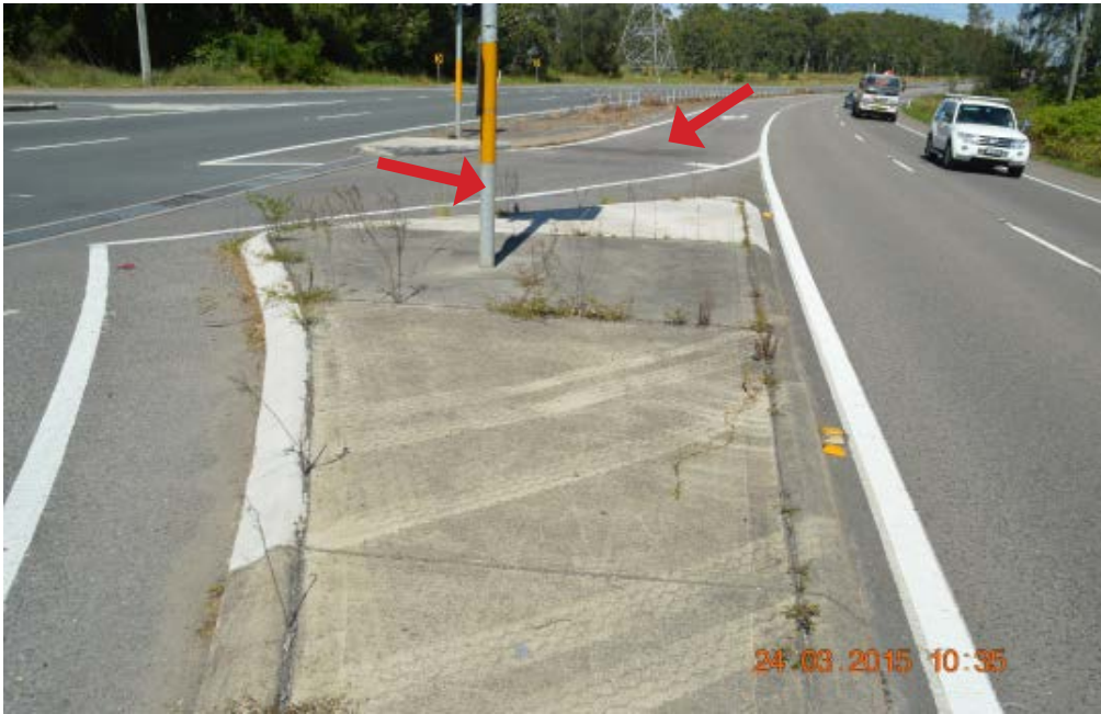
General view of the west side of the Pacific Highway at 100 metres to the south of the 'Slippery When Wet' street sign on the north side of the intersection with Old Punt Road.
