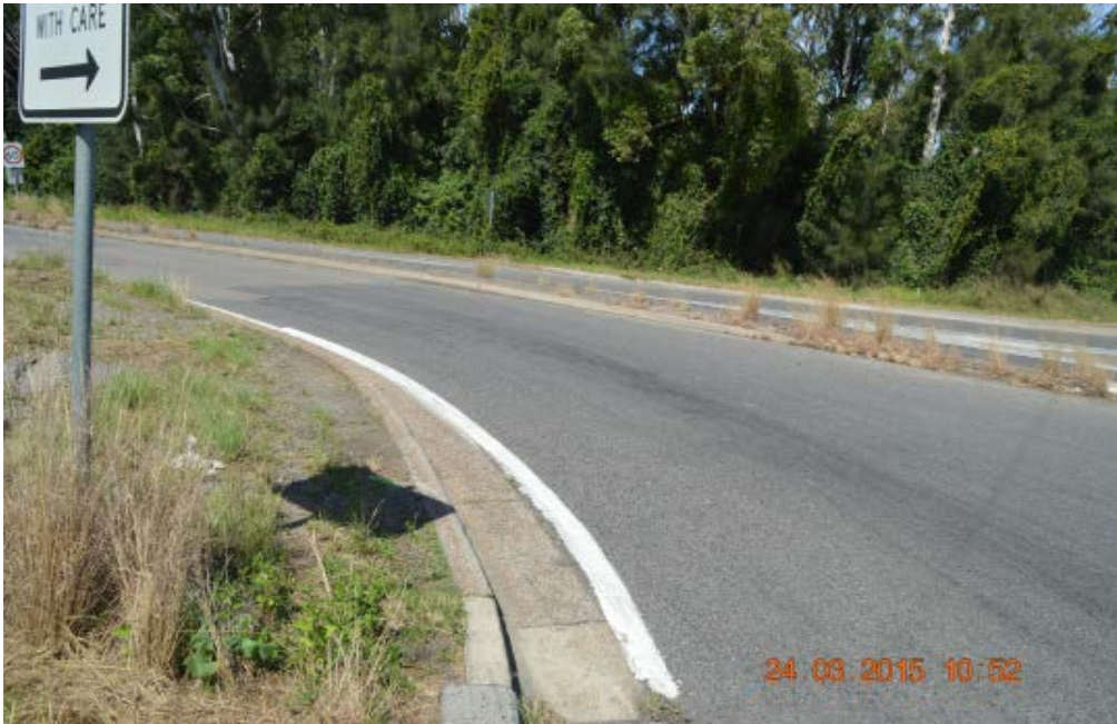
North side of Old Punt Road at 10 metres from the intersection with the Pacific Highway.
