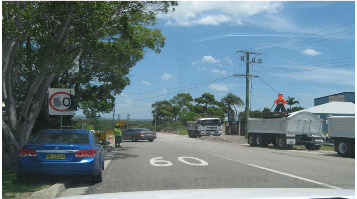
PHOTO P51 View South in Old Punt Road to Road Construction Site.
