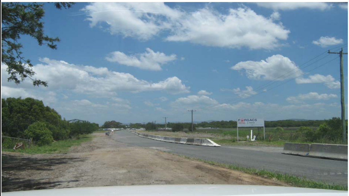
PHOTO P54 View South Along Old Punt Road South of Laverick Ave. Pipe Storage Behind Tric Lok Barriers on Right.
