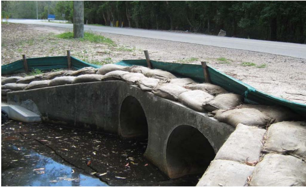
PHOTO P37 View of Upstream Headwall in twin 1050 Dia. RCP Culvert at Ch 2100
