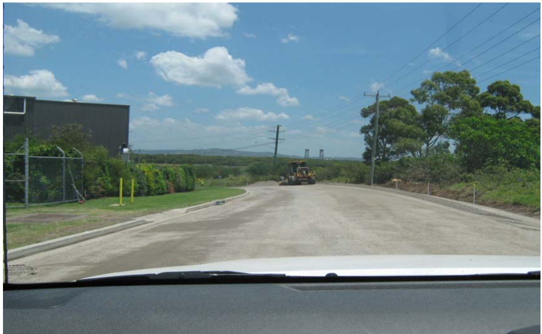
PHOTO P52 Section of Reconstructed Old Punt Road. Asphalt Surfacing required for Completion.
