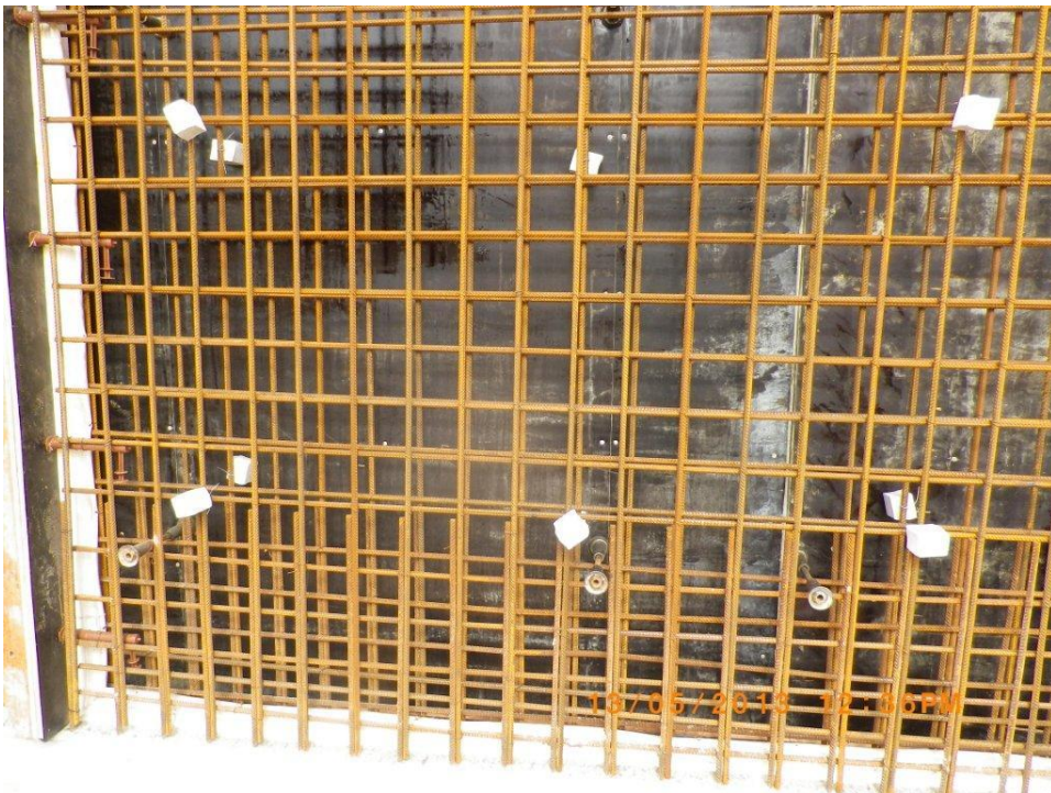
Waterstop at base and side of wall.
