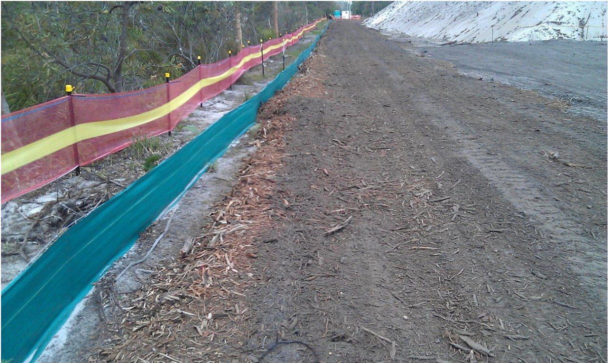
Access Track with sediment fence and barrier fencing. Mulch used to stabilise access tracks.
