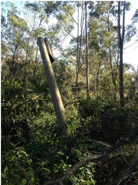
Box and pole (No. 77) fallen over due to storm damage
