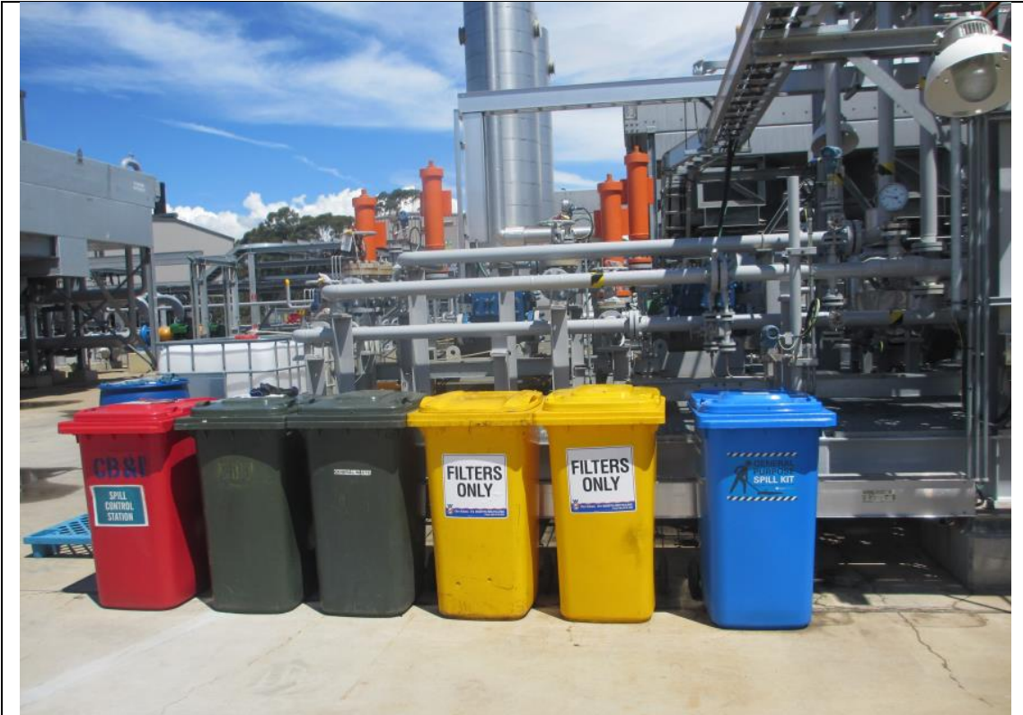
Photograph: 7 Amine filter bins, general waste bins and spill kits located in the process area
