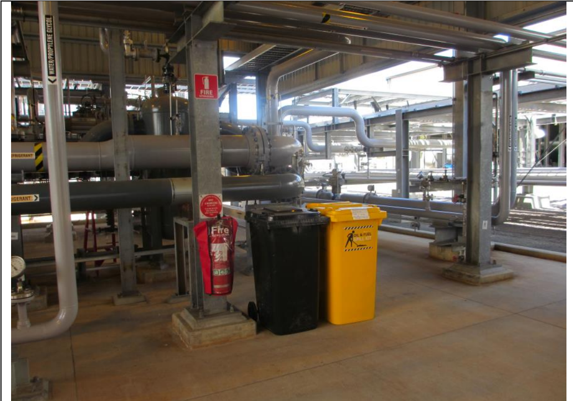
Photograph: 9 | General waste bin and spill kit located in process area
