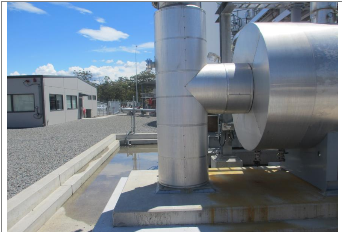
Photograph: 6 Leak of propylene glycol from amine reboiler – contained within bund
