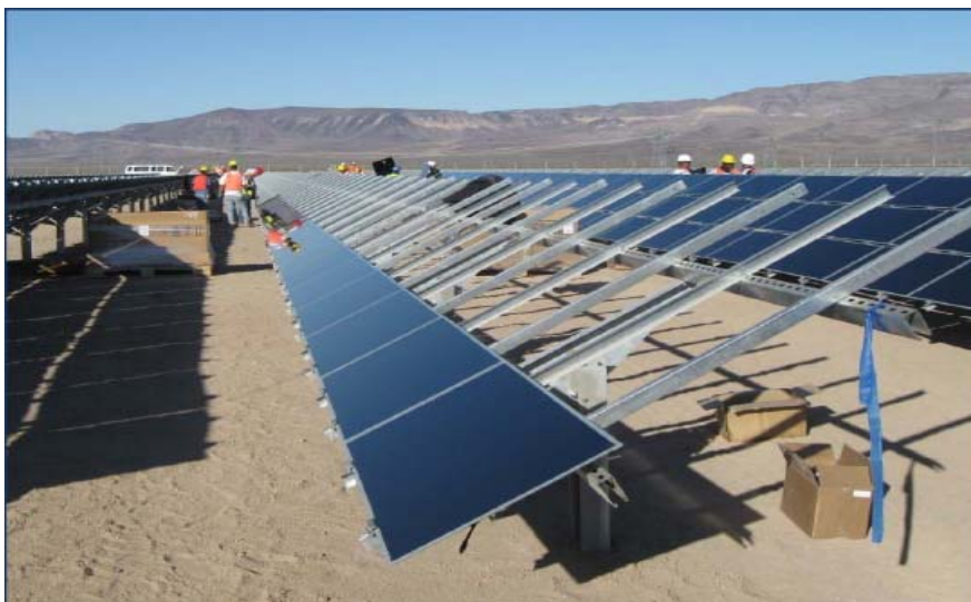
Figure 3-3 First Solar modules and racking tables.
