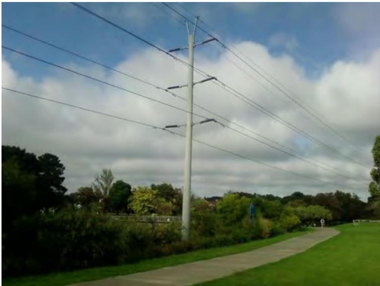
Figure 3.3 Example on left of spun concrete poles and wires (image provided by AGL)
