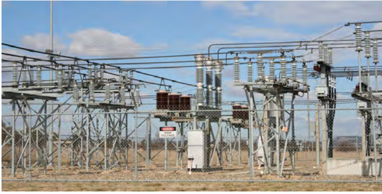
Figure 3.2 Typical substation found in Australia
