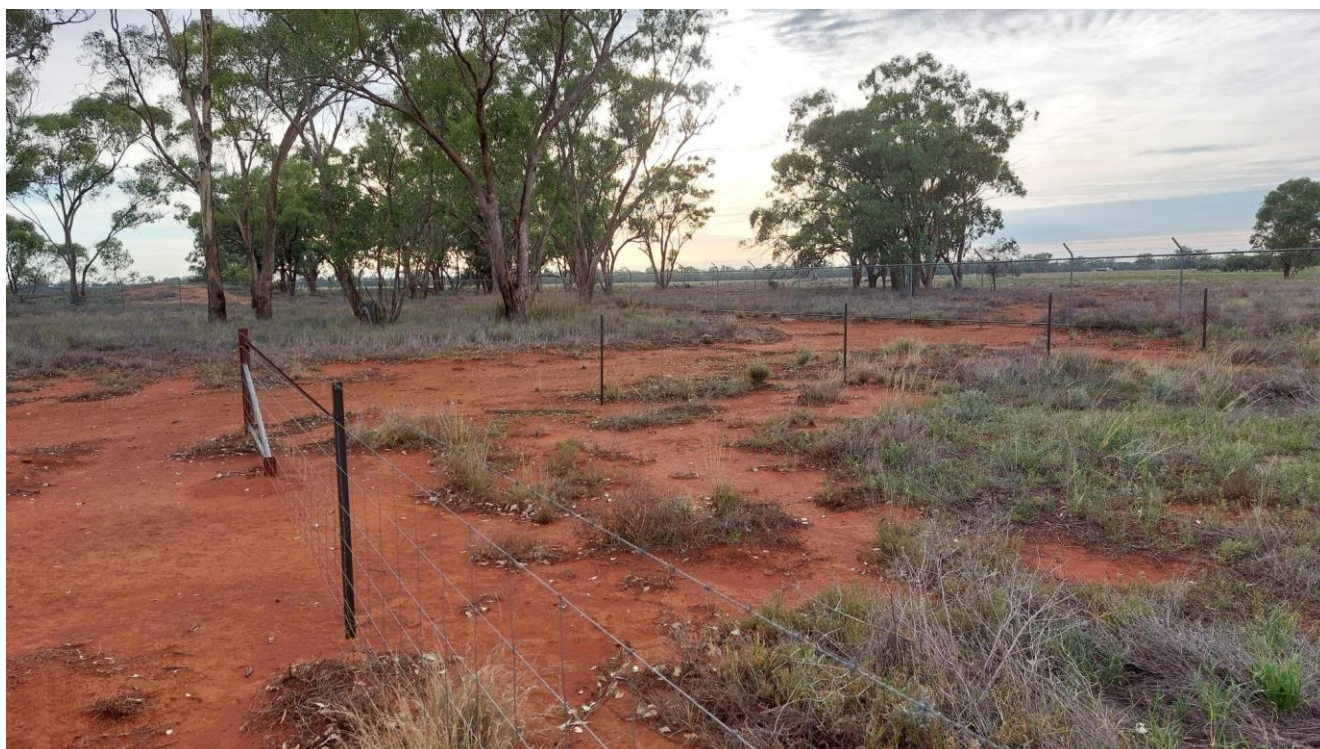
Plate 19. Existing fence condition looking east along the eastern revegetation area (January 2024, Year 7)
