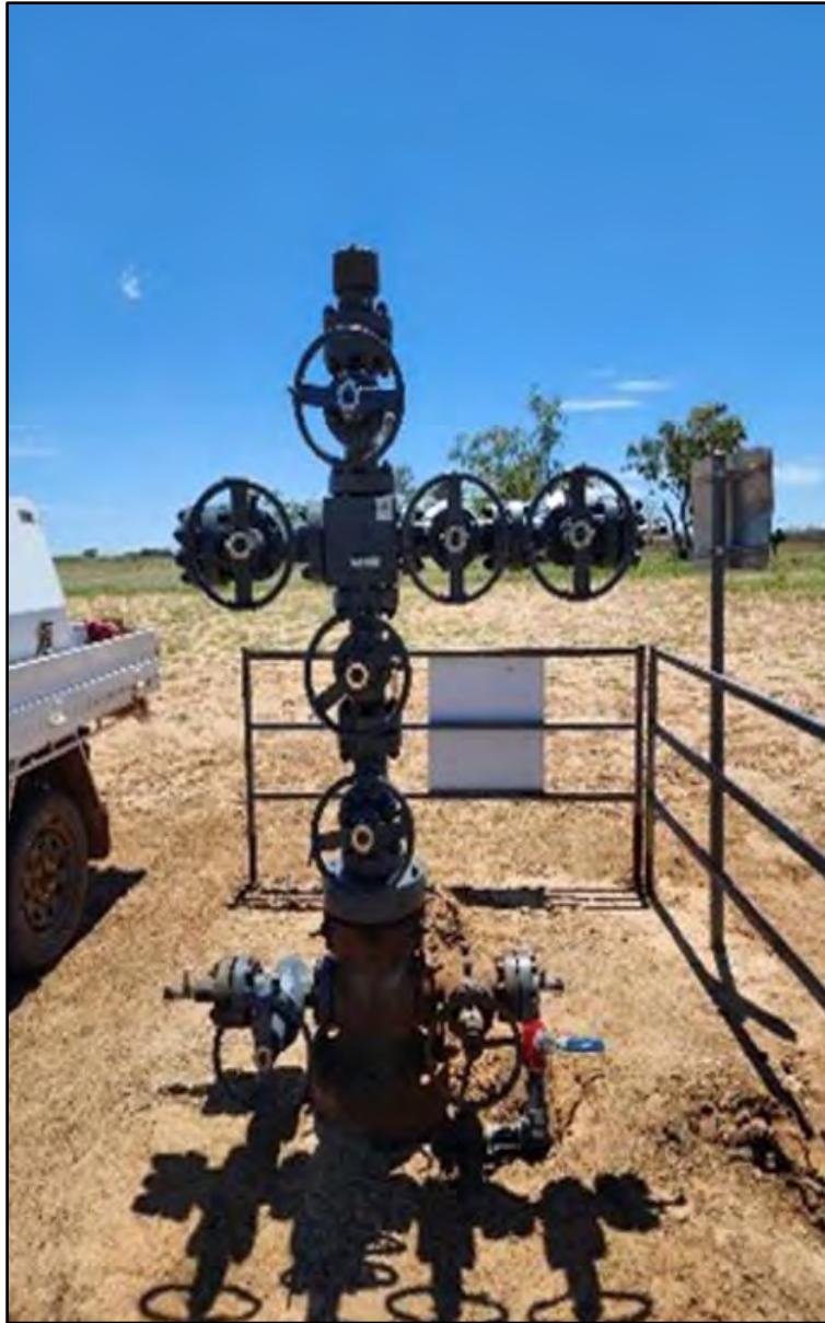
Figure 2-2. Wellhead of West Noorindoo 1 (AGL, 2023b)
