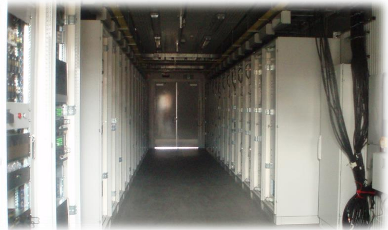
Control, protection and metering panels inside SSB
