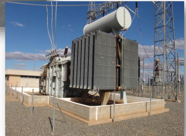
Typical bunded transformer at 220/22kV
