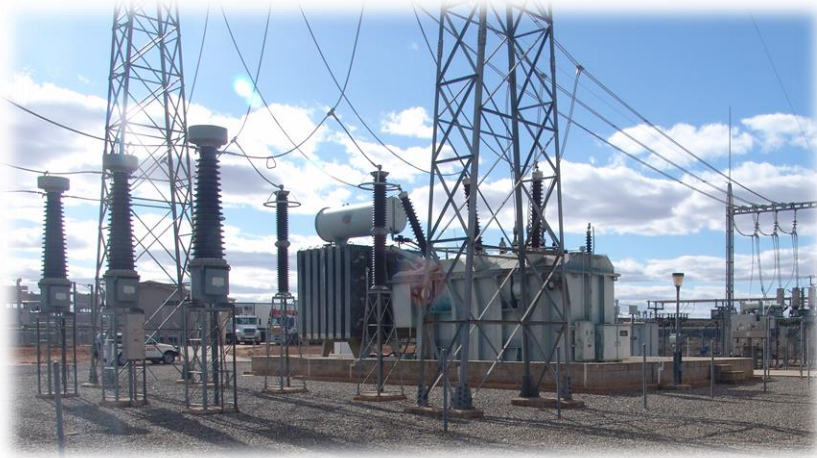
Typical 220kV switch bay
