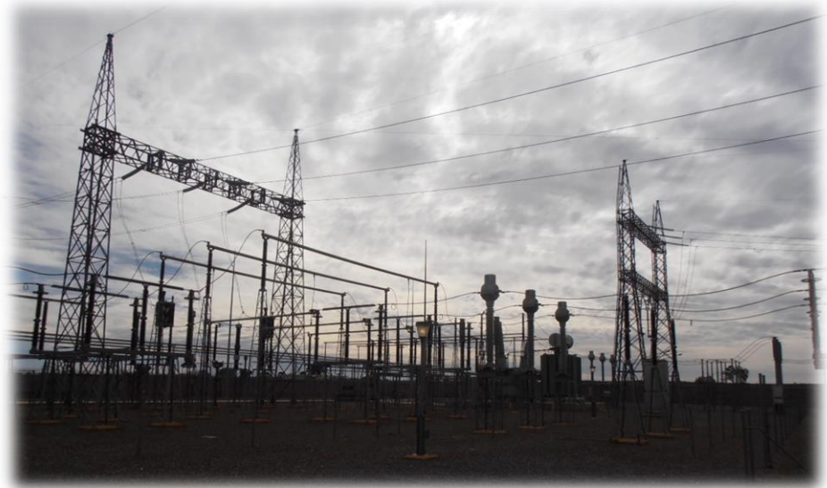
TransGrid's existing Broken Hill 220kV Substation.
