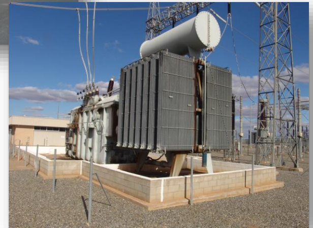
Typical bunded transformer at 220/22kV
