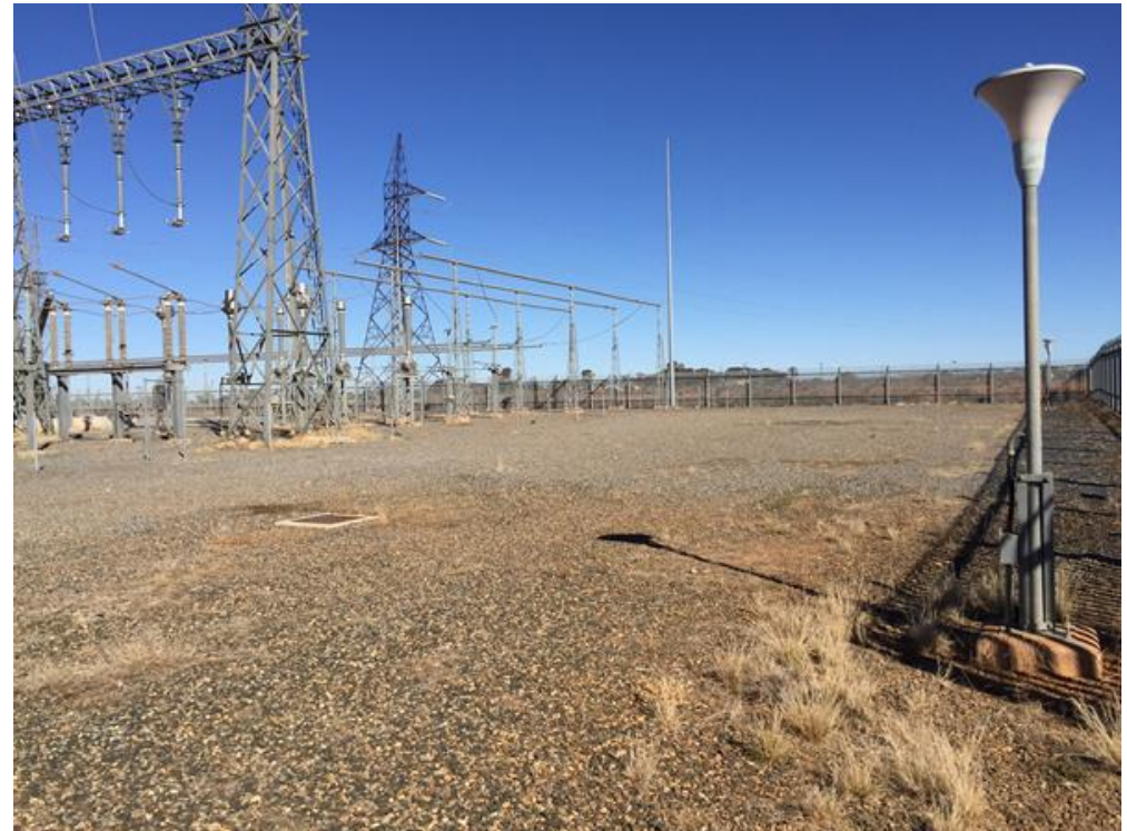
TransGrid's existing Broken Hill 220kV Substation.
