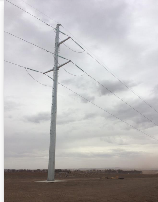
Typical 220kV Transmission Line Single pole, single circuit arrangement.
