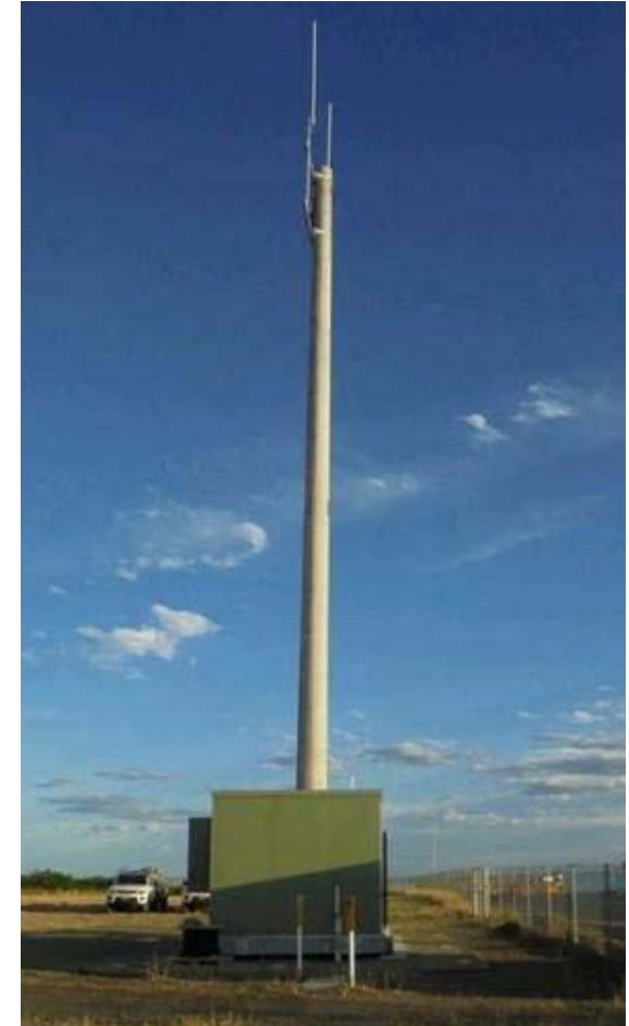
A typical 20m monopole with an omni antenna configuration
