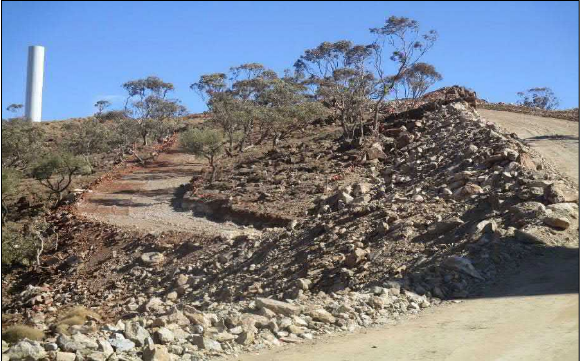
Photo: Underground HV electrical trench between T34 and T35 (Area 7): Bench to be retained and rehabilitated to minimise disturbance to Porcupine Grass Sparse Woodland.
