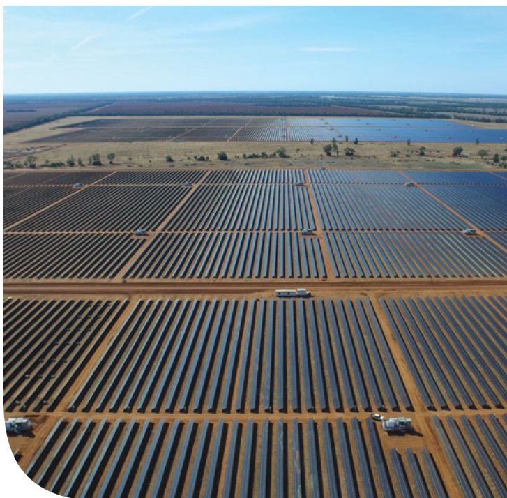
AGL's 102 MW solar plant in Nyngan, New South Wales
