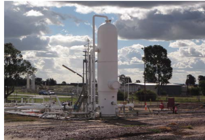
Wallumbilla LPG Plant
