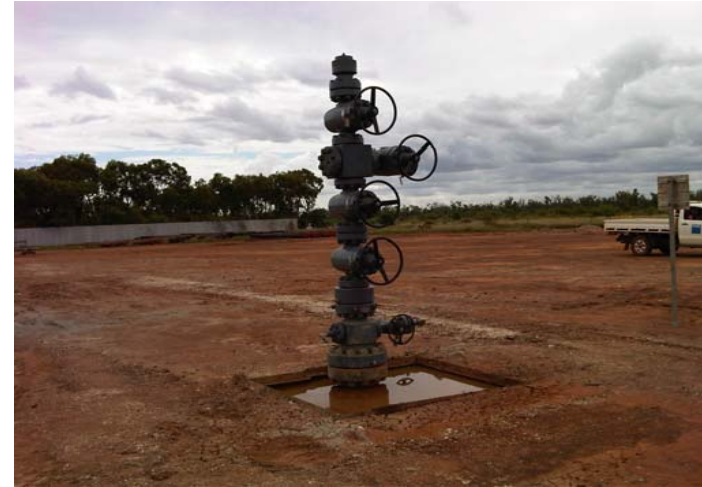
Injection well - Silver Springs 12
