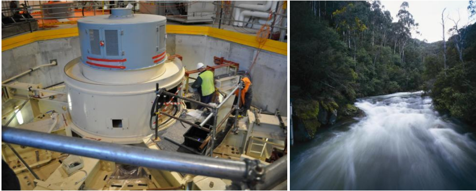
Hydro power station
