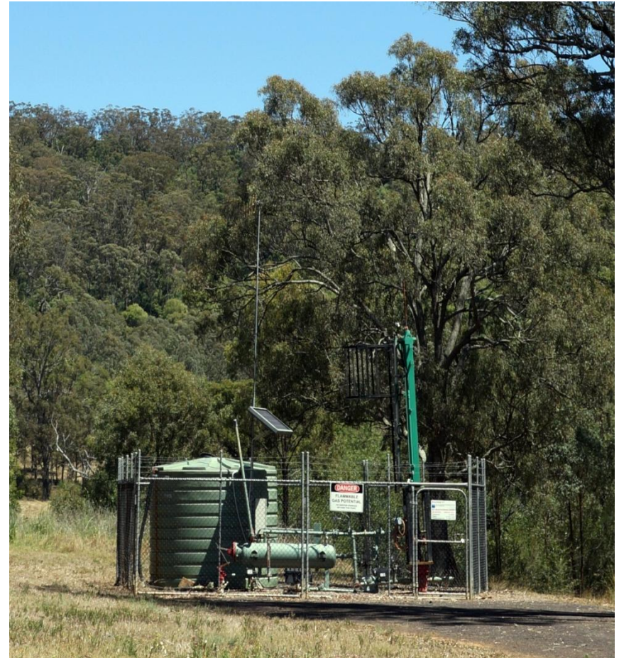
Camden gas well
