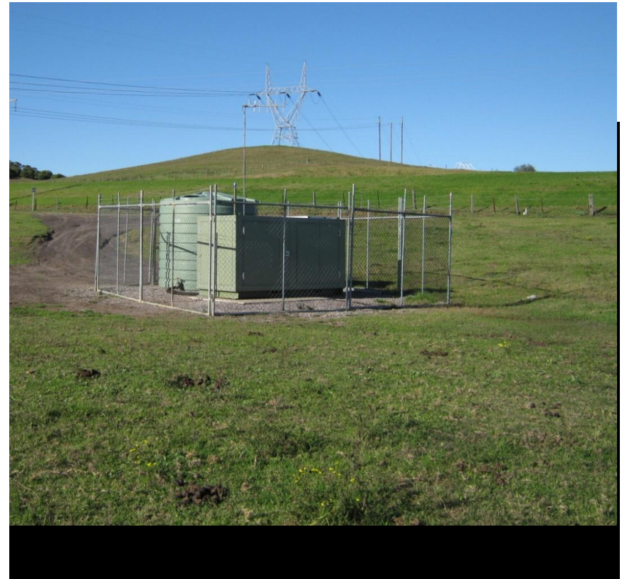
A CSG well in the Macarthur region
