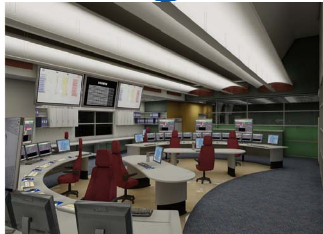
Modern control room (AGL Torrens)
