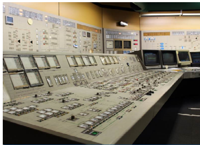
Bayswater control room
